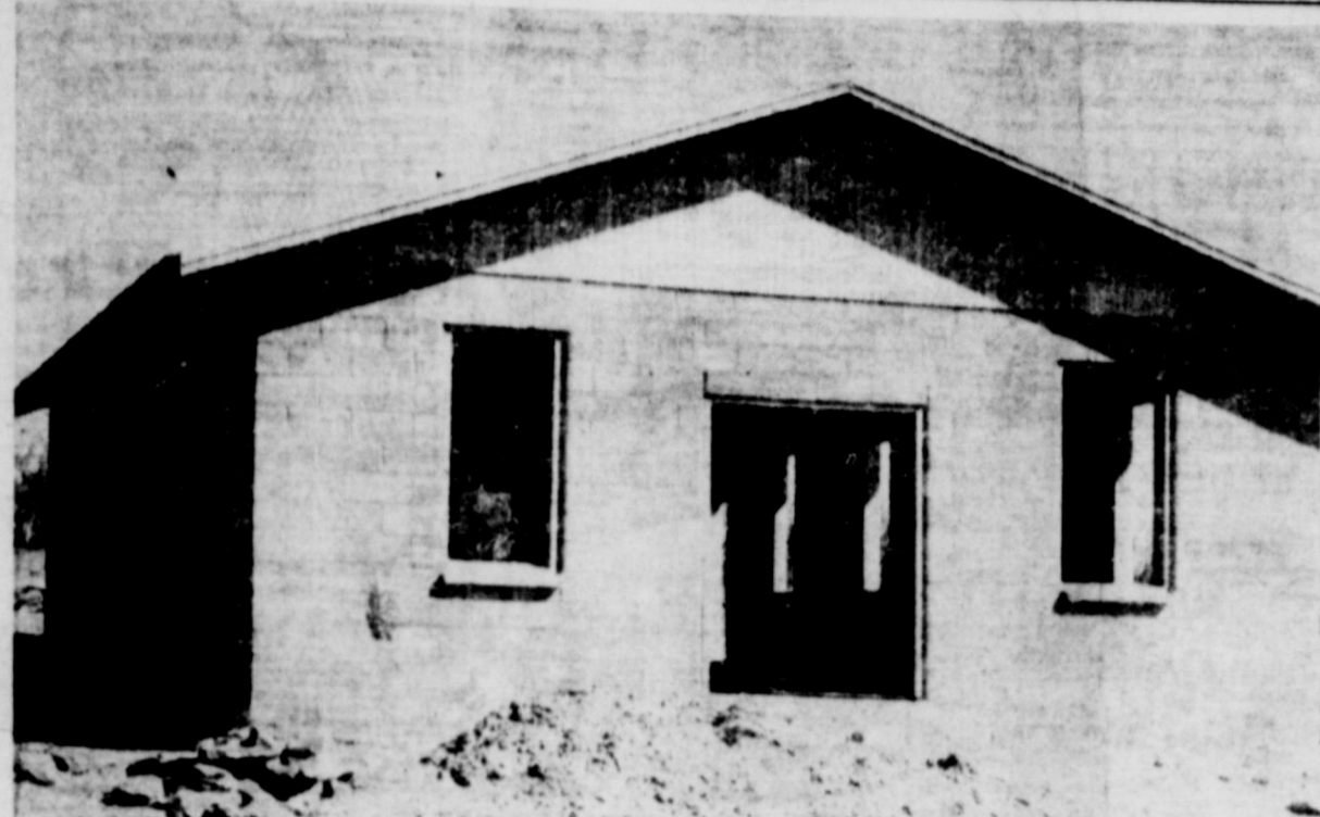
NEW NIMROD CLUBHOUSE . . . Pictured above, the new clubhouse of the Nimrod Neighbors Progress Club, now under construction. Work on the building is expected to be completed this week and an open house program is planned for the public next Monday night. The building measures 25 x 50 feet and will house a meeting room, kitchen, rest room and storage closet, built at an approximate cost of $2,000.00. Review staff photo.
