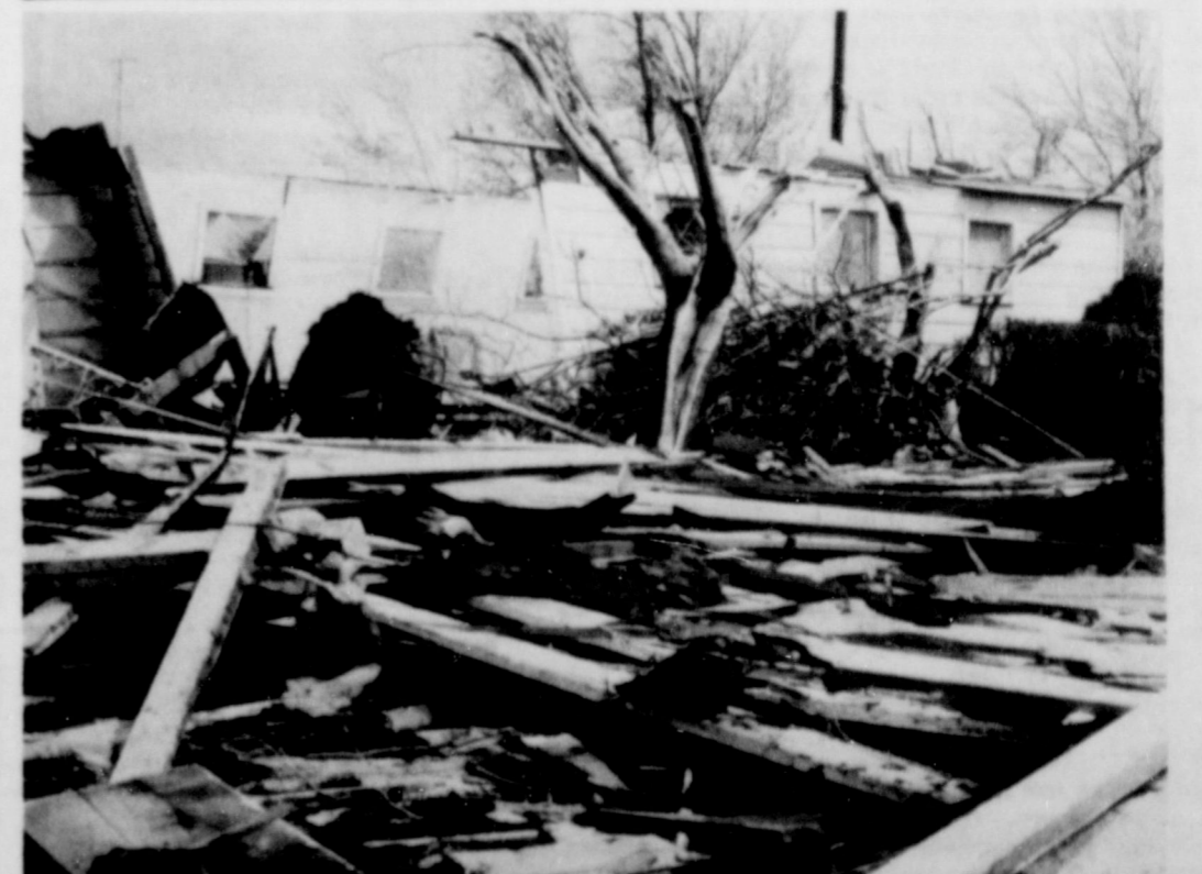
STORM'S AFTERMATH... Twisters did millions of dollars in damage, both in Hereford and in the Lazbuddie area in the early morning hours Monday. The above scene is just off Star Street in Hereford, one of the hardest-hit sections, showing a house that was completely demolished.
