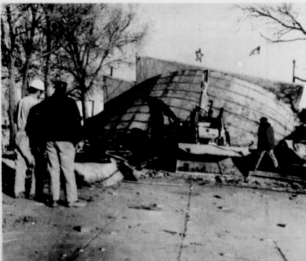
LANDMARK RAZED... The old quonset building at the corner of Eighth and Main Street was torn down this week by City of Friona employees. The old building, which has been empty for a number of years, at various times has housed an Oliver dealership, garage and blacksmith, and machinery storage.
