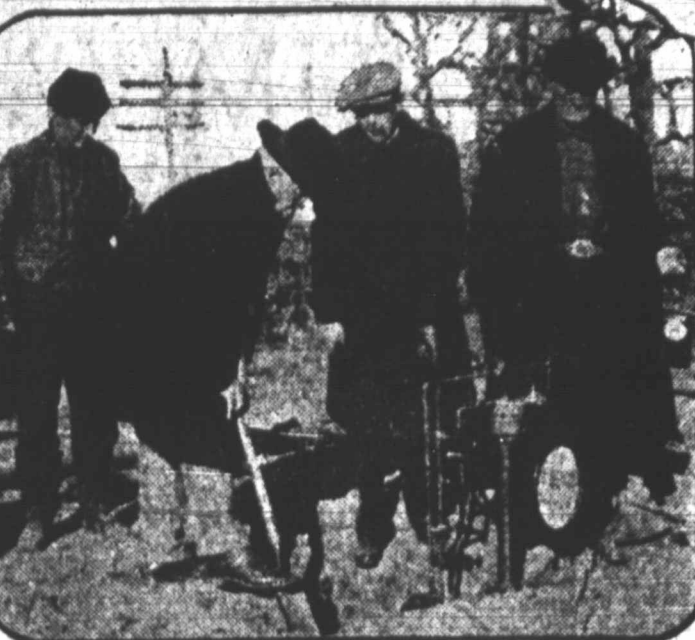
Cold weather and low gas pressure constitute a civic emergency, according to Mayor W. B. Nicodemus of Drumright, Okla. So he gathered a committee of citizens and tapped a private main for general supply. Picture shows the committee at work, with the mayor second from the right.
