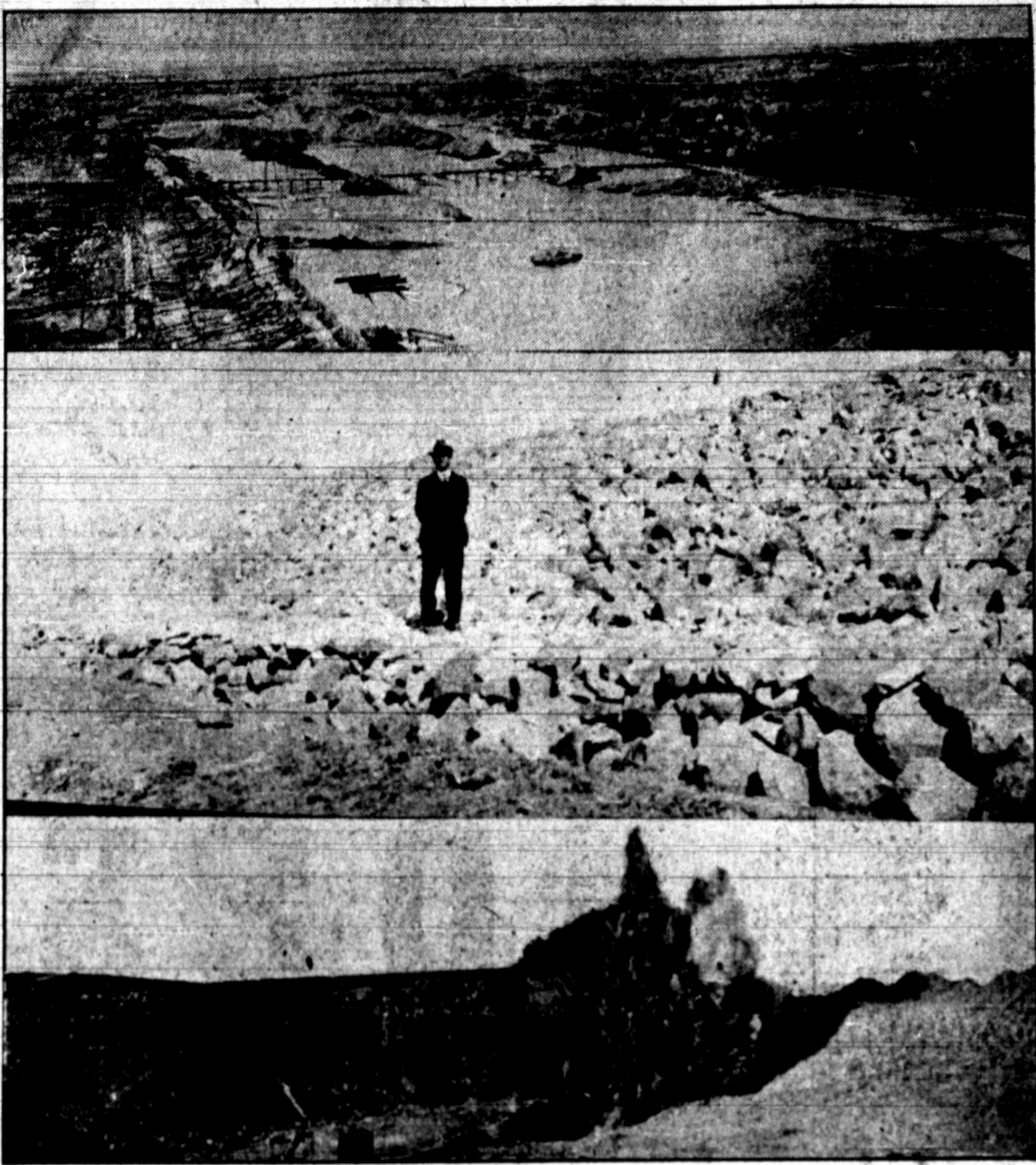
The top picture shows the progress of the dredge, on the gorge dam, which structure is now nearly 40 feet above the river bed. The water shown in the picture is drained back into the pool in which the dredge works, and is used over and over again. The dredge operates in such a way that the water drains toward the center line of the dam, carrying with it the impervious clay that will form the core of the completed structure. The second picture shows the rip-rap construction on a completed portion of the embankment. The heavy rocks are laid in such a way as to minimize the action of the water on the up-stream face of the dam. J. L. Lockridge, resident engineer, appears in the picture. The evening "strafe" at the site of the service spillway is shown in the bottom picture. This is one of the many shots set off each evening as the 20-foot excavation goes deep.
