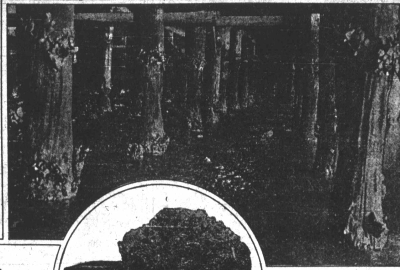
Wharf at Charleston, S. C., being destroyed by "shipworms"
