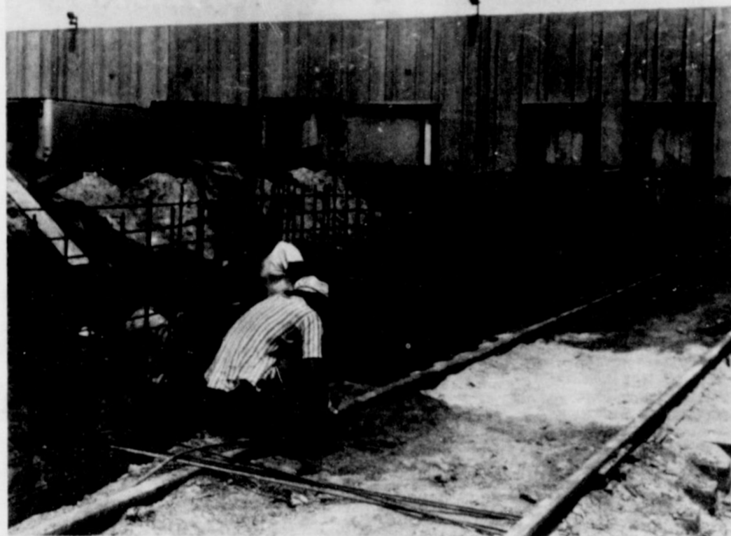
CONSTRUCTION. . . Part of the construction which is underway in Friona can be seen in the above photos. The upper photograph shows the apartments being constructed on West Ninth Street by the Medlock Company of Lubbock. Four of the project's six tri-plex apartments have been framed, and work is proceeding at a good pace. Below is a scene at Missouri Beef Packers' Friona plant, where the 60,000-square foot addition for the plant's breaking facilities is underway.
