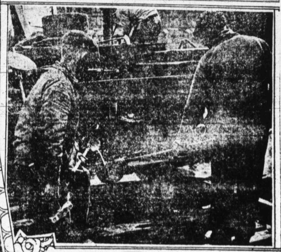
DRAWING OFF MOLTEN LEAD TO BE POURED BETWEEN PLATES AT THE JOINTS TO MAKE THE CONTACT PERFECT
