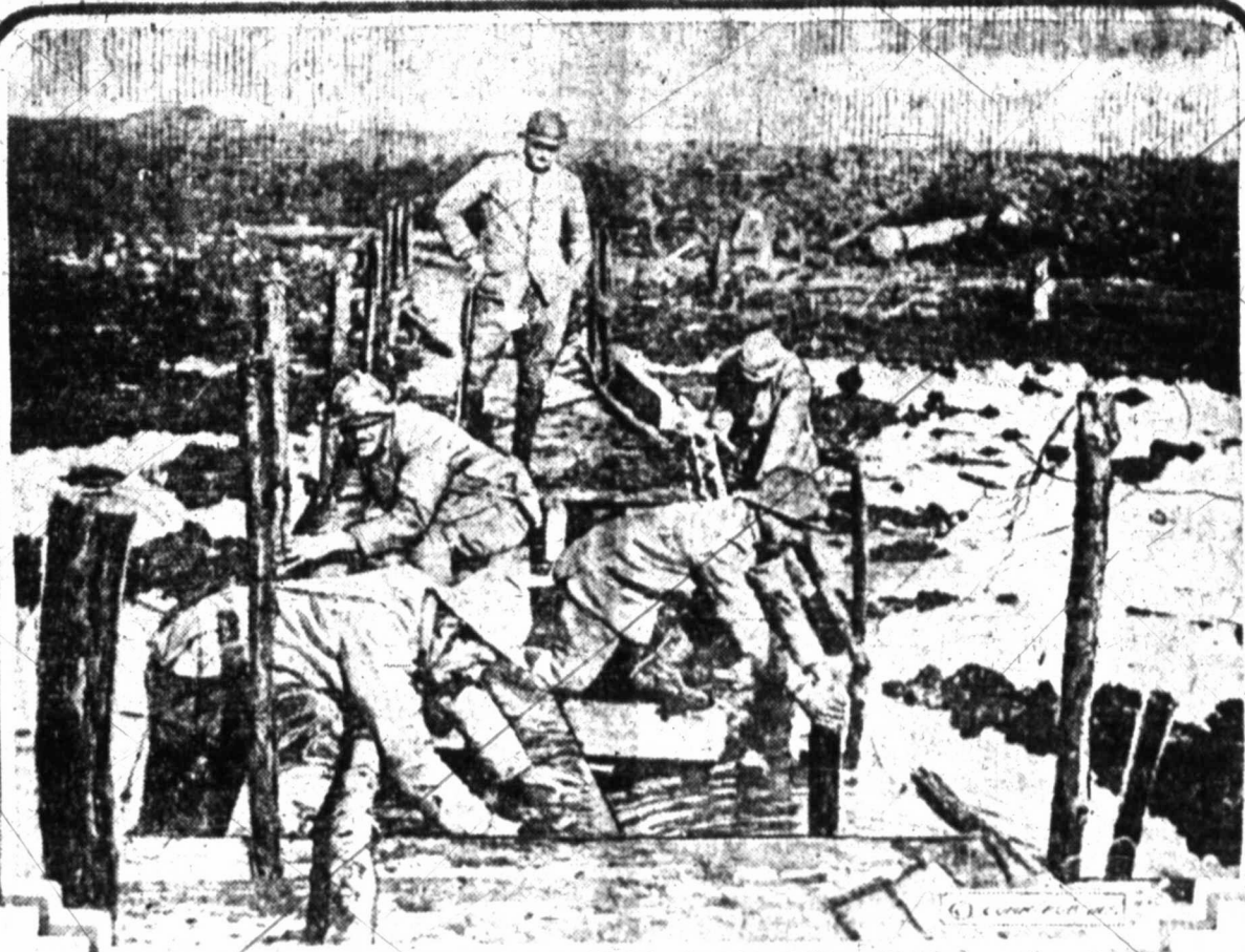
French engineers are constructing a foot bridge over a bit of low ground in Belgium. The bridge, looking in its present state rather insecure, will support, when completed, a battalion of men. Shell holes in this low ground are frequently from twenty to thirty feet deep and filled with water.
