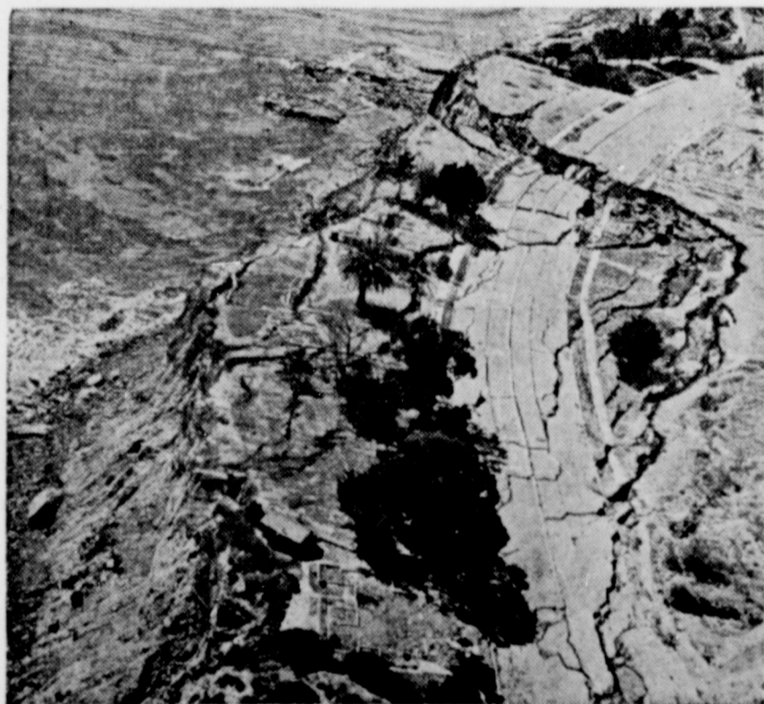
New cracks radiated out from the chasm which girdles the six-acre bluff at Point Fermin, Calif., which is slowly slipping into the ocean. Houses situated on the bluff were removed to safety several months ago.
