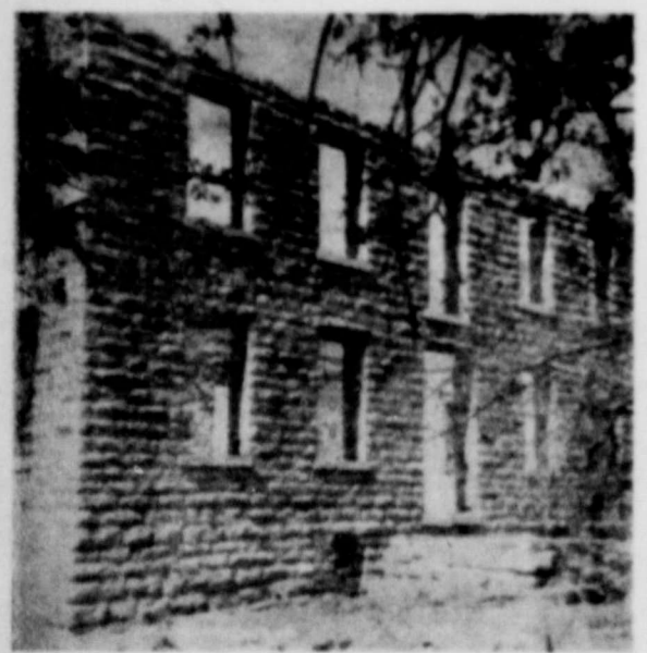
STURDY AND STRAIGHT are these native rock walls, which have withstood 80 years of exposure to the weather. A close-up of the mortar between these hand-quarried rocks reveals that it is still serving its purpose well and has crumbled in very few places. This view is from the front of the house, which faced the old road when the house was built. Since then, a new road has been built below the hill, this one discontinued.
