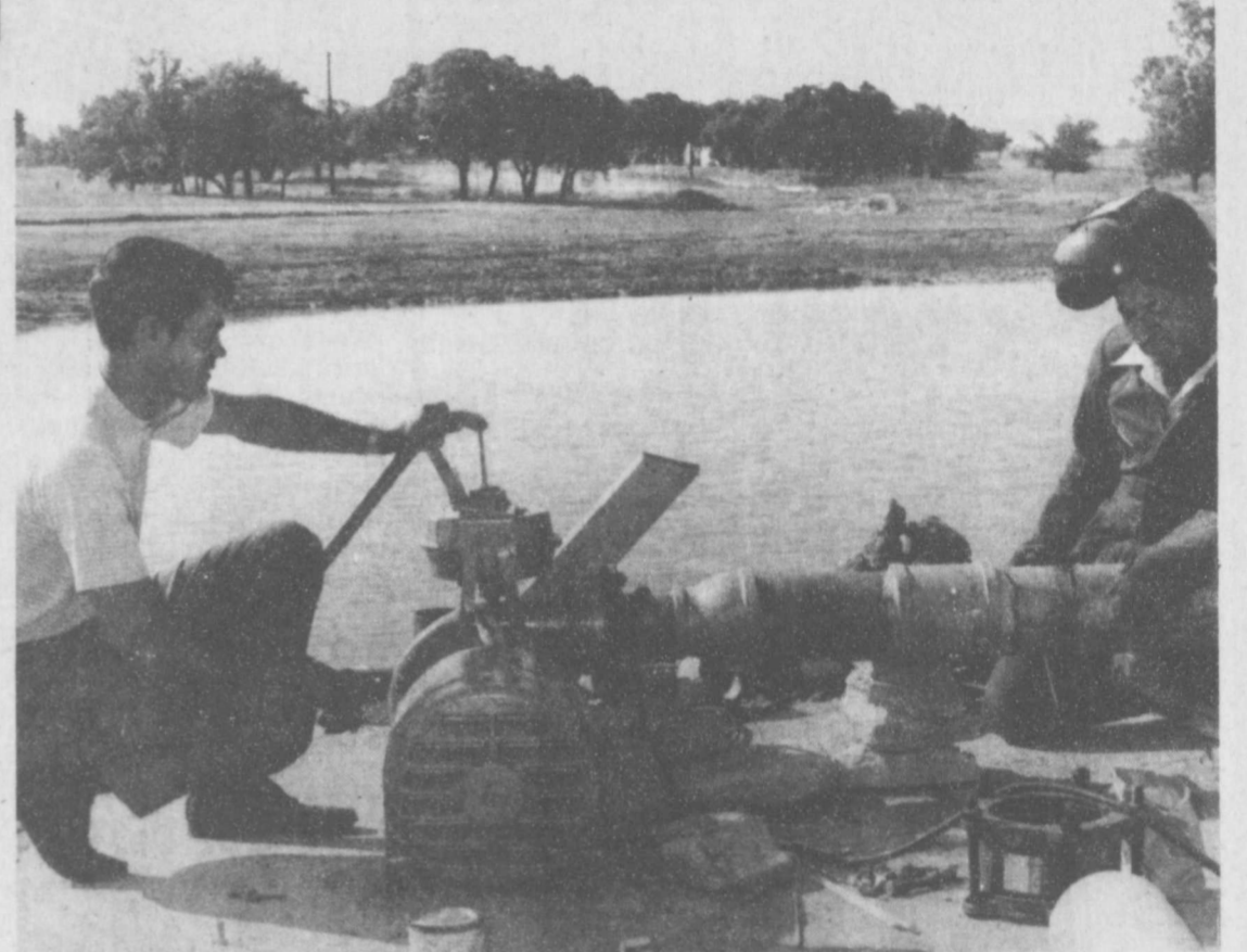
Club Pro-Manager Dave Schackelford watches as Horley Whaley welds a joint of pipe to the water pump that will be the heart of the Gatesville Country Club irrigation system. The system will go into service this week.
