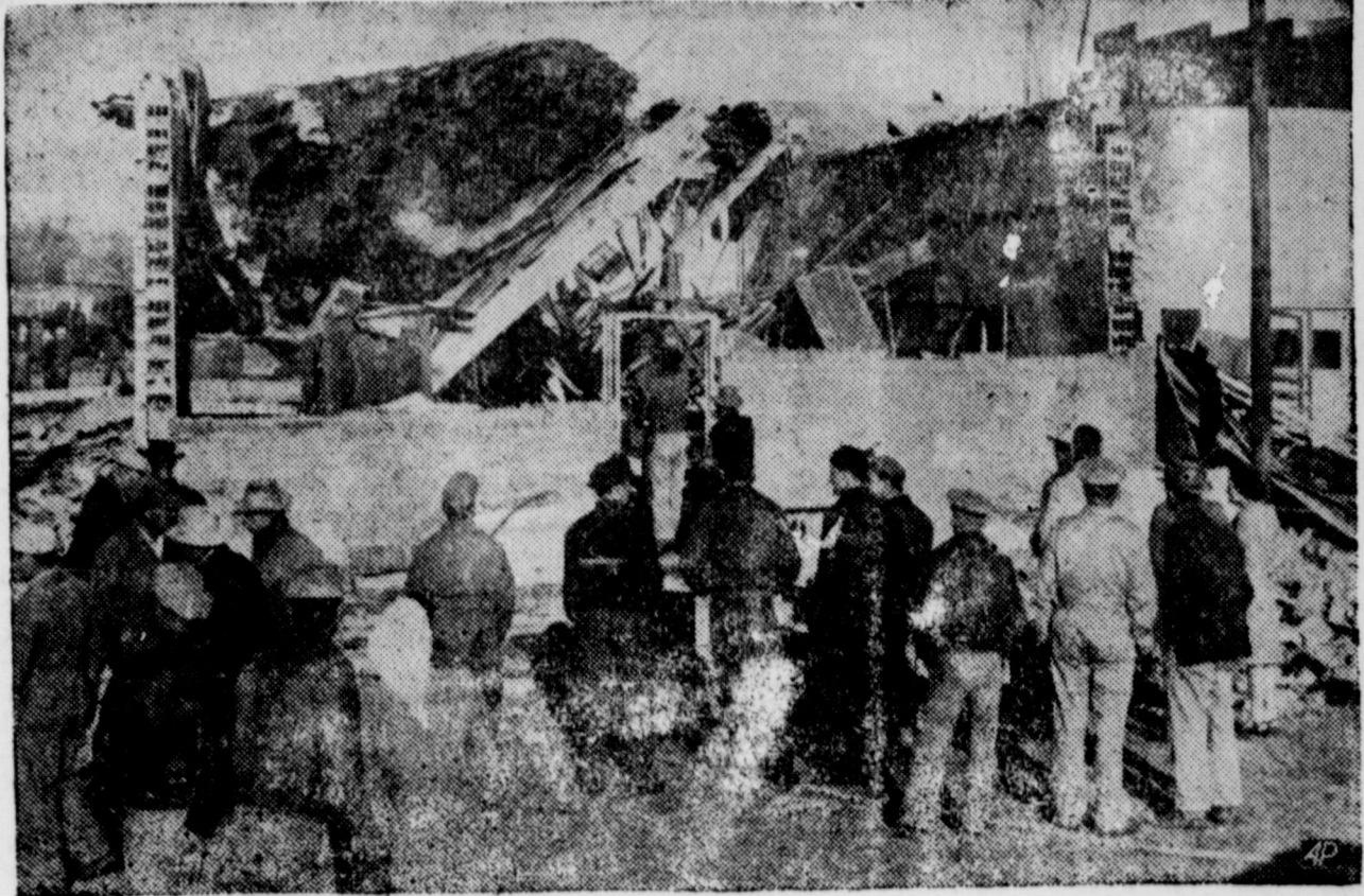
An explosion heard four and a half miles away wrecked the brick postoffice (above) at Mulehoe, Texas, sending five persons to the hospital, including postmaster A. J. Gardner. The explosion occurred when Gardner knelt to light a stove (AP wire photo)
