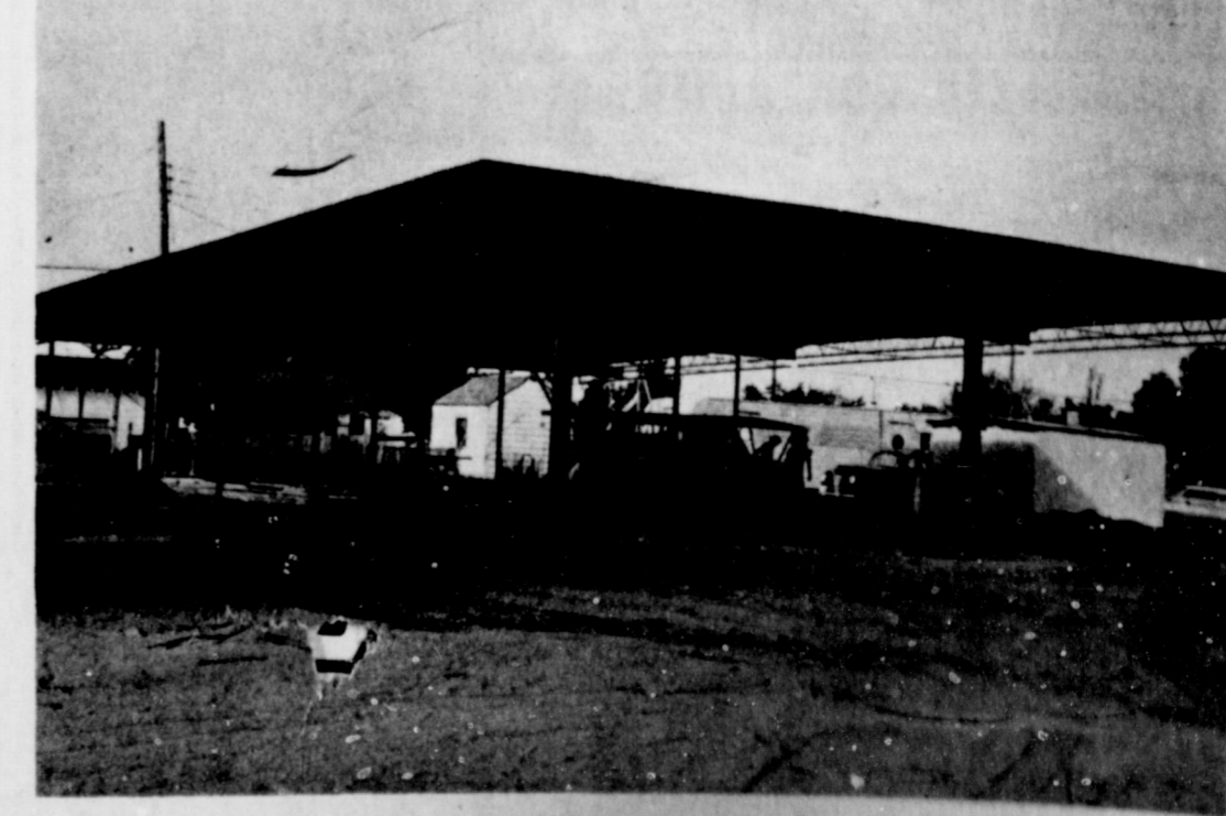
DAIRY QUEEN UNDER CONSTRUCTION...Construction on the new Dairy Queen at Twelfth Street and American Blvd. is going quite rapidly with the inner structure nearing completion this week. The new family dining place is due for an opening around the first of October. The Dairy Queen will feature a drive-up and walk-up window plus a dining room that will seat 60 people.
