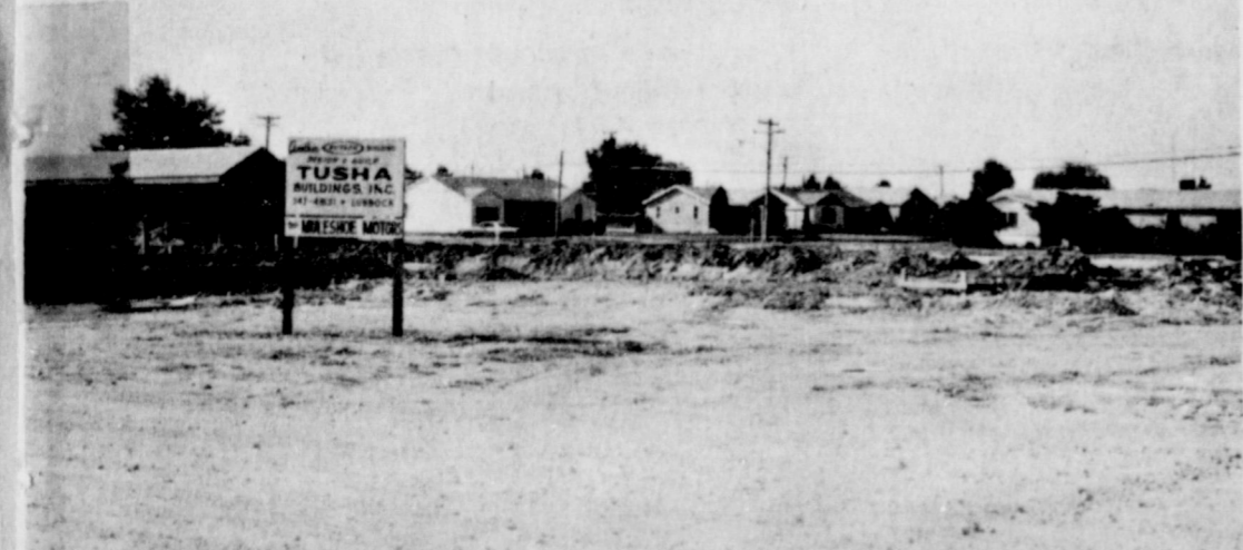
CONSTRUCTION ON NEW FORD HOUSE PROGRESSING...Construction on the new Muleshoe Motor Company building is progressing with the foundation being dug and laid this week. The building is due to be finished by the first of the year.
