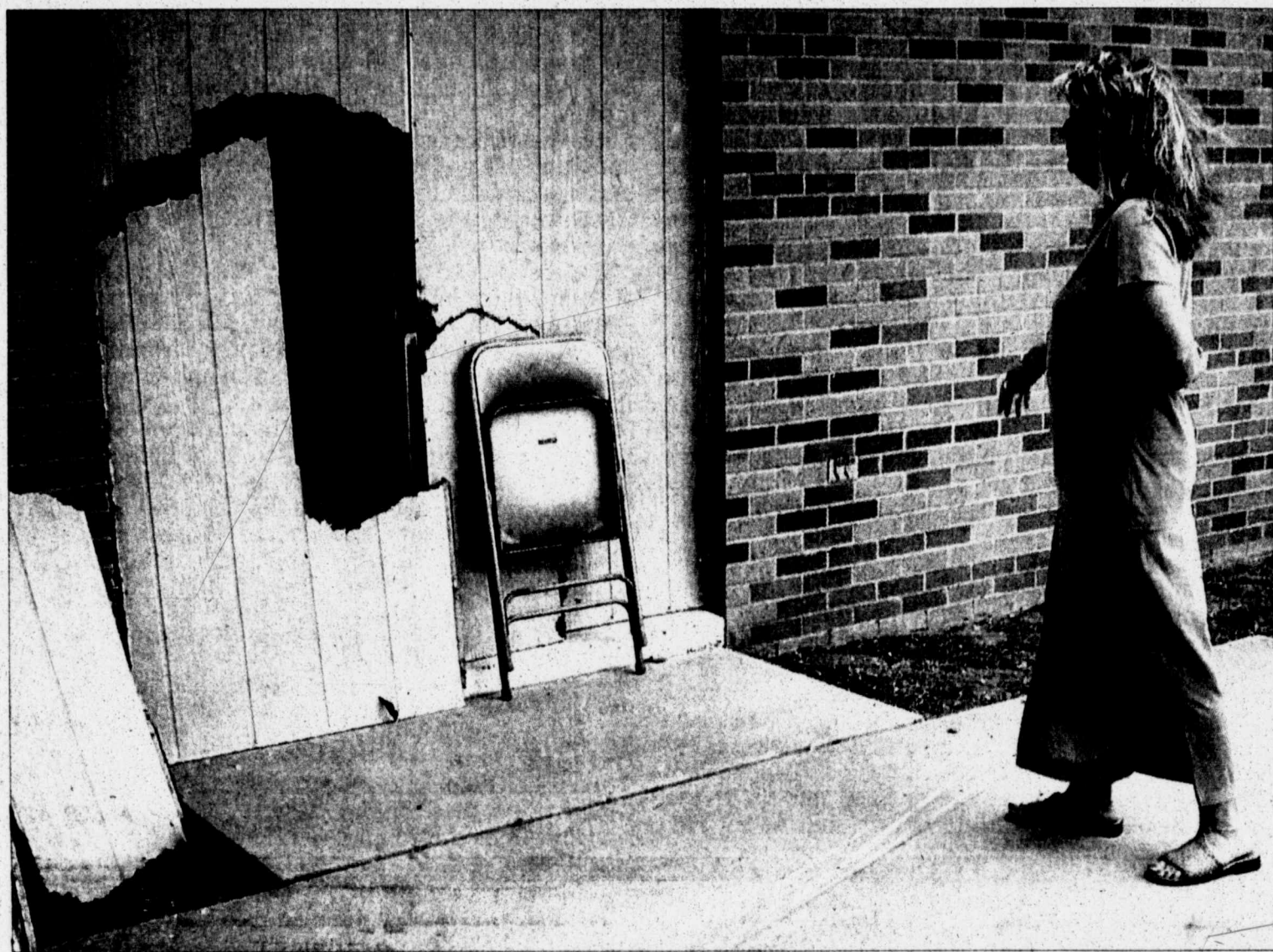
Shann Thomas, director of Victim Services of Big Spring, inspects damage to the agency's building on Airbase Road Monday morning. Victim Services has been burglarized twice in the last three weeks.
