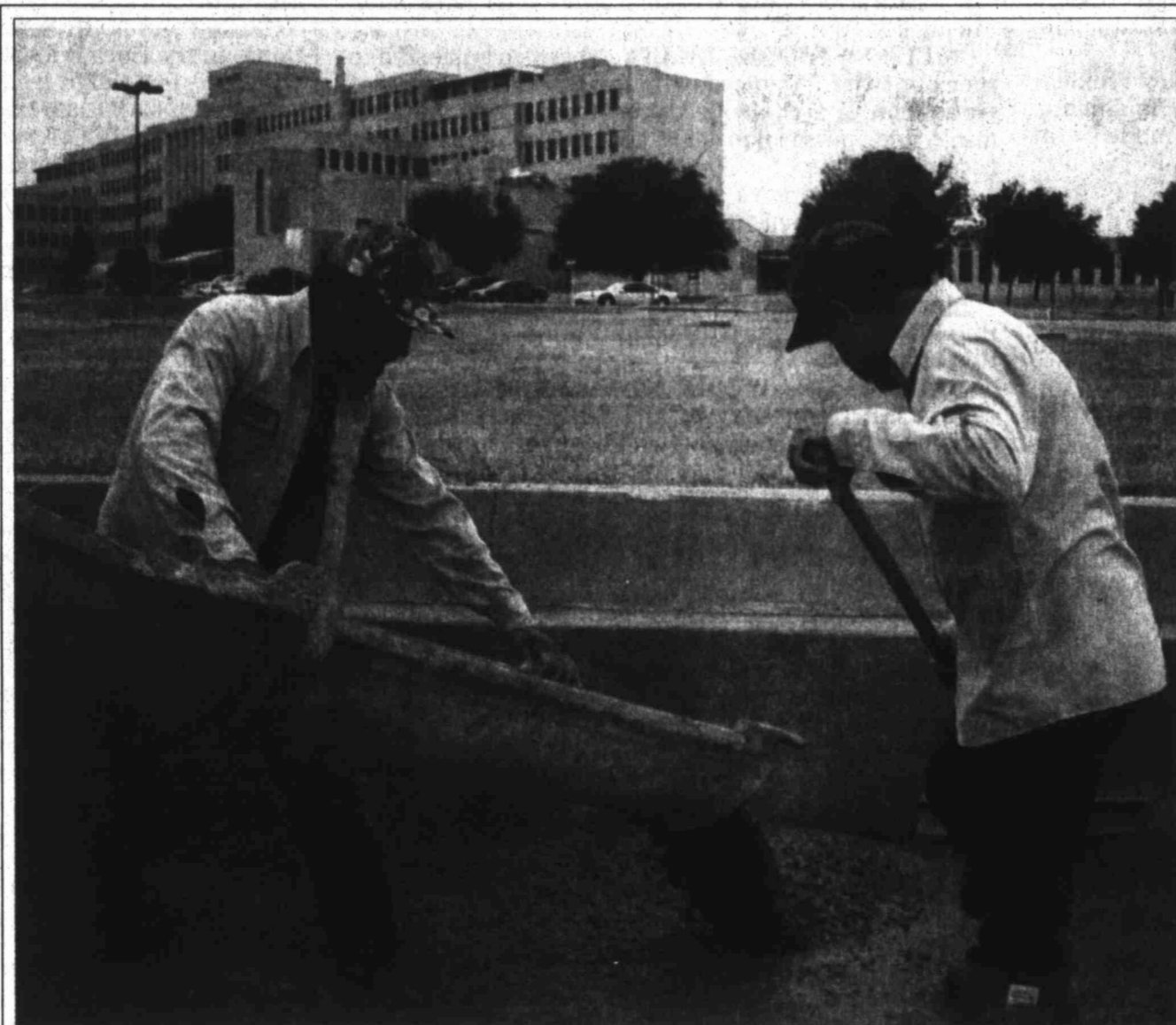
City of Big Spring employees Jorge Parra, left, and Raul Martinez lay concrete provided by Big Spring business Transit Mix Tuesday morning to create a sidewalk along Gregg Street in front of the VA Medical Center. The work is part of a project between the hospital, city and the Texas Department of Transportation to spruce up the area in front of the hospital.
