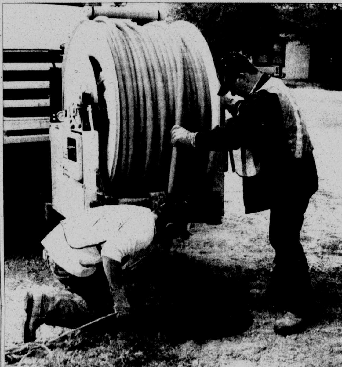
HERALD photo/Thomas Jenkins City employees Randy Roach, right, and Justin Denton work on jetting a sewer main on 16th Street Monday afternoon. City Water Distribution and Collection Superintendent Rick Boiles said his department experienced a high number of sewer-related calls Monday.
