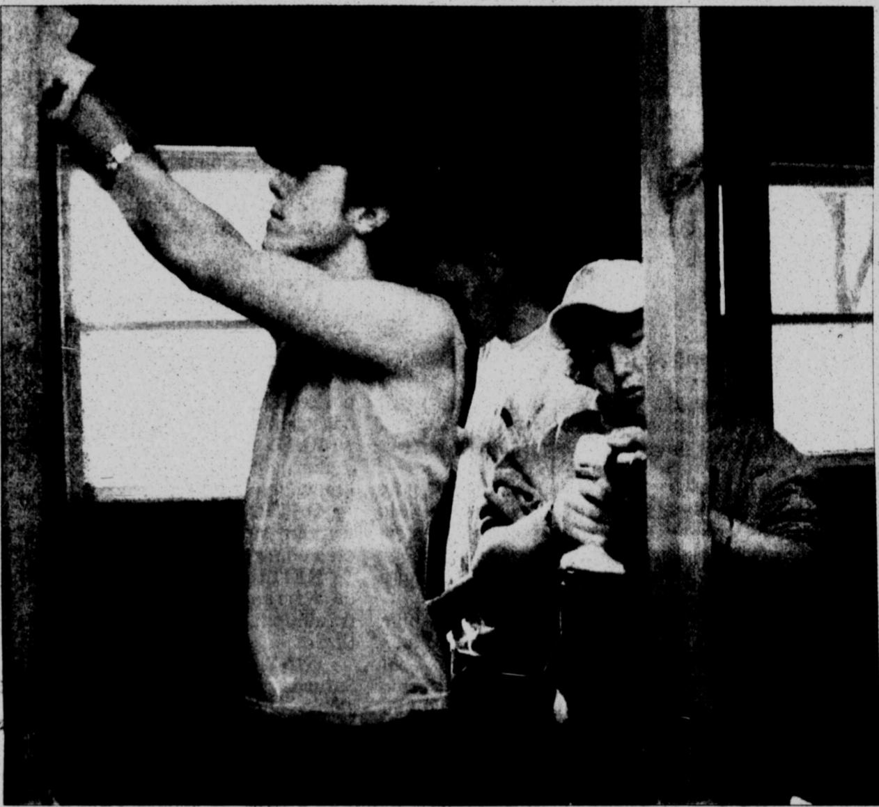
Community of Hope First Church of the Nazarene youth members Branden Burchett, 16, left, James Geraldson, 18, and Lance Gross, 14, help renovate the House of Hope, a project to turn a house on Scurry Street into a temporary home for pregnant women.
