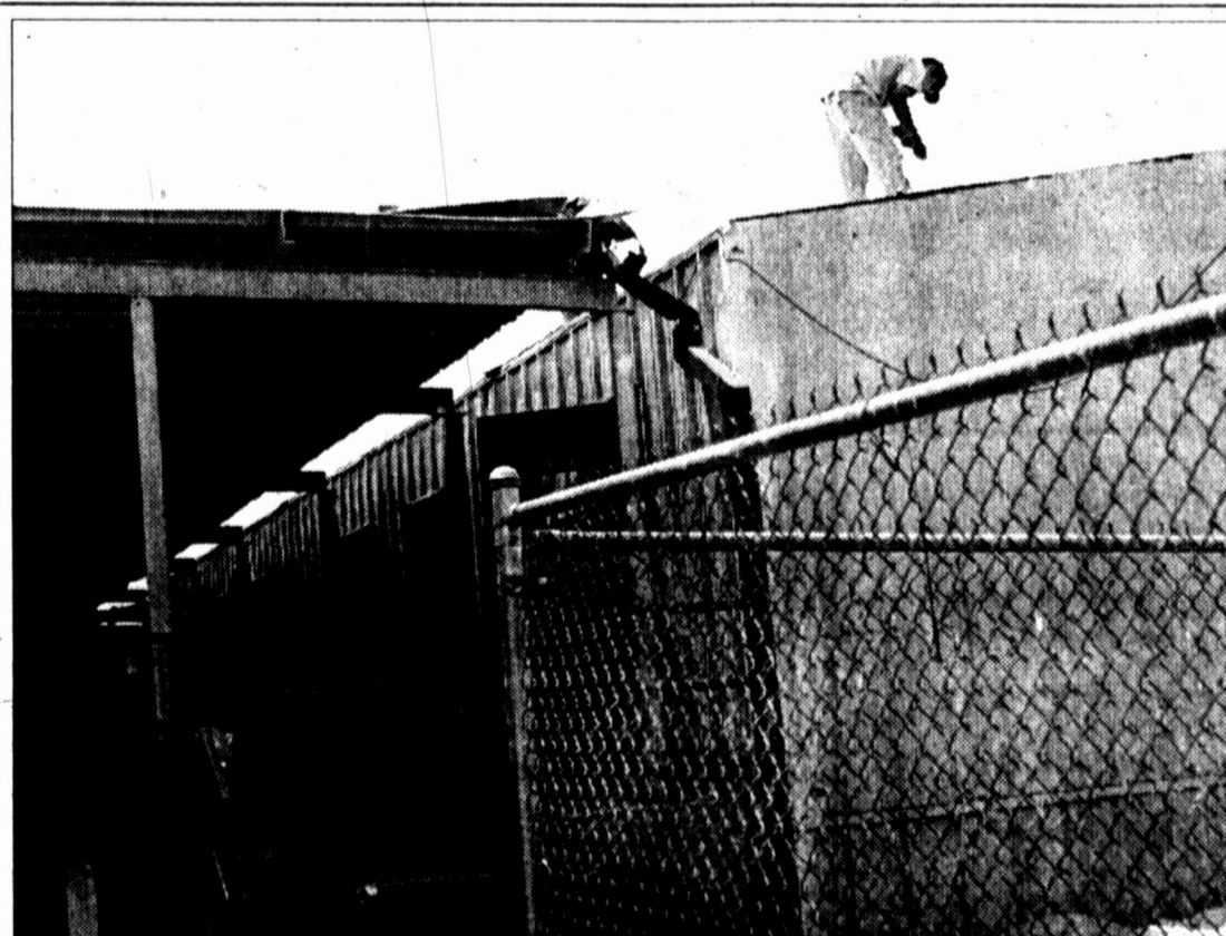
HERALD photo/Lyndel Moody An employee for Johnston Construction of Big Spring repairs damages to the roof of one of Moss Elementary's portable buildings. Strong gusts Monday night ripped the roof off the building, causing $10,000 in damage.
