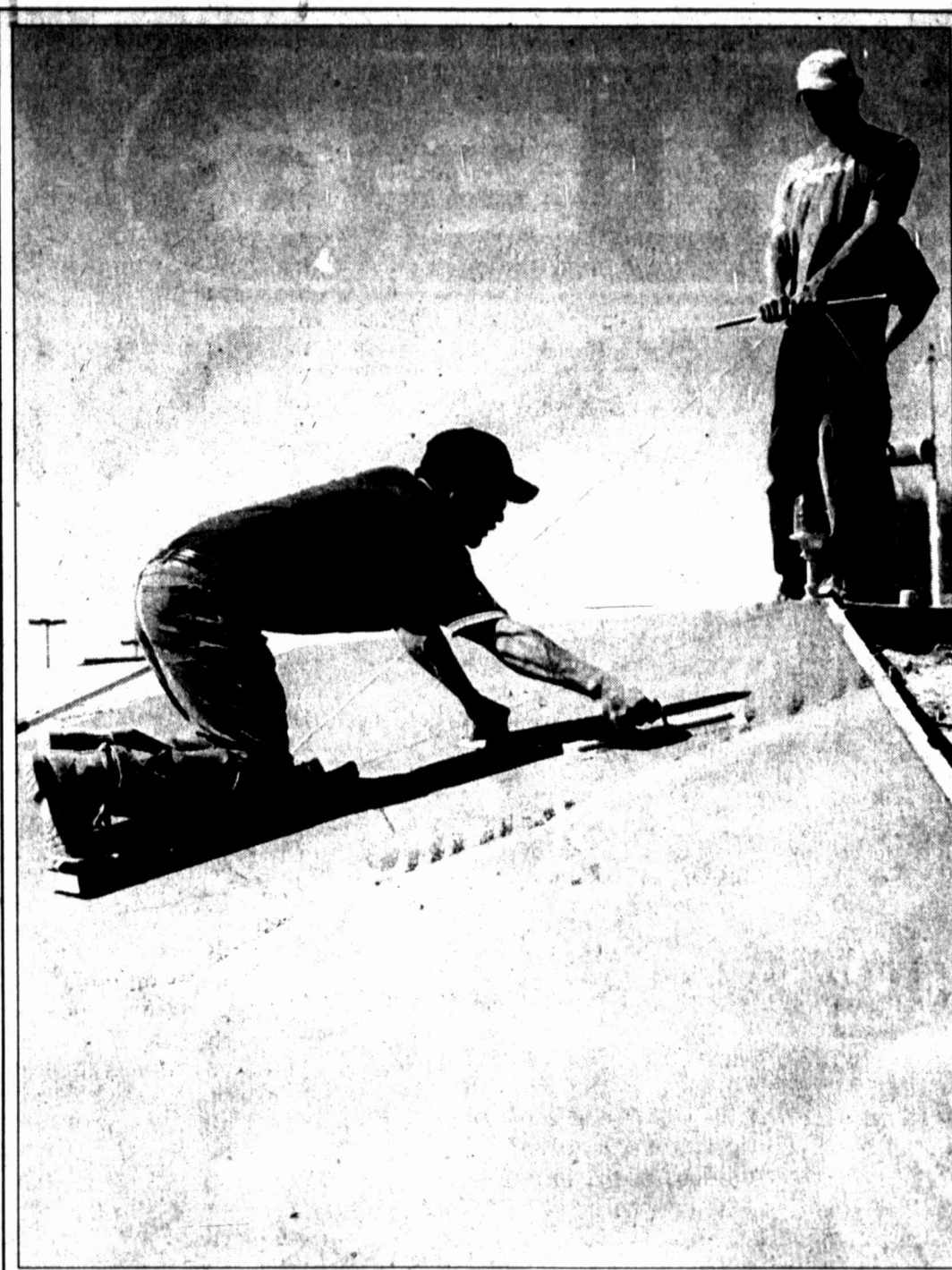
Workers smooth concrete in the process of constructing a helipad at the VA Medical Center. HERALD photo/Tommy Wells
