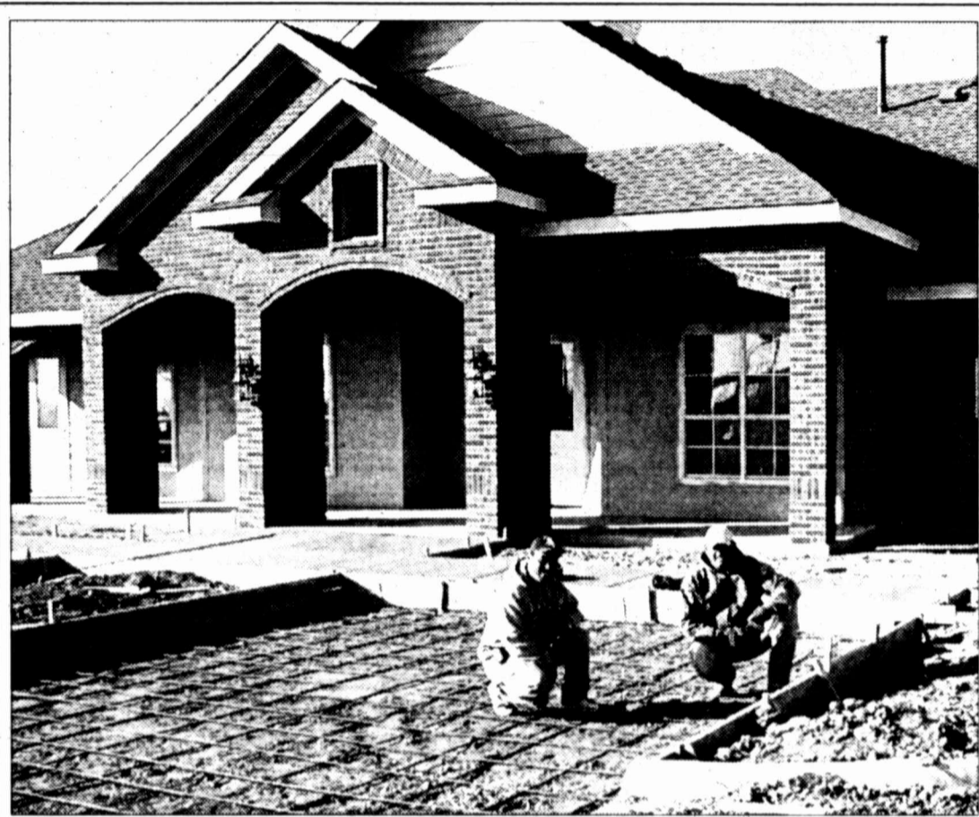
HERALD photo/Roger Cline Limestone Ridge resident David Sandoval and concrete contractor Joe Natividad examine preparations for pouring the parking lot for the clubhouse at the income-controlled apartment complex. Although only about half the buildings are complete, several of the apartments have already been leased.
