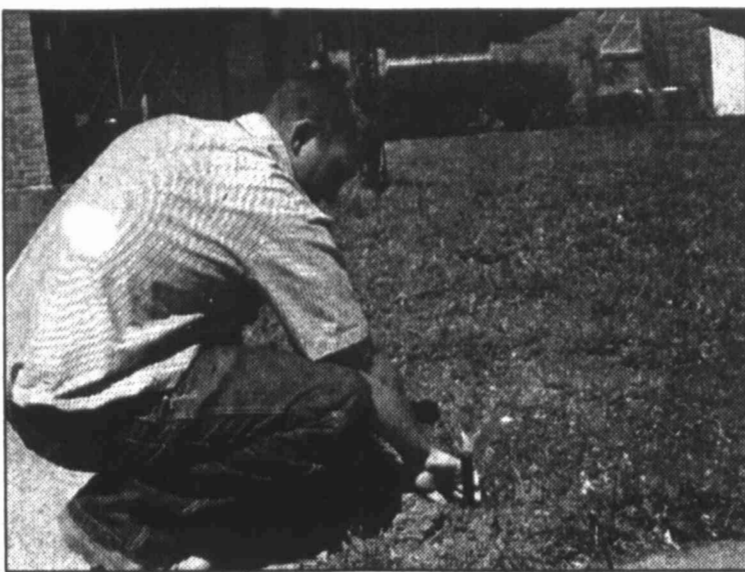
HERALD photo/Lyndel Moody Culligan employee Cory Cook adjusts a water sprinkler head. Richard Wright, the owner of Culligan, also owns Wright Sprinkler Systems, which offers irrigation system installation and repair.
