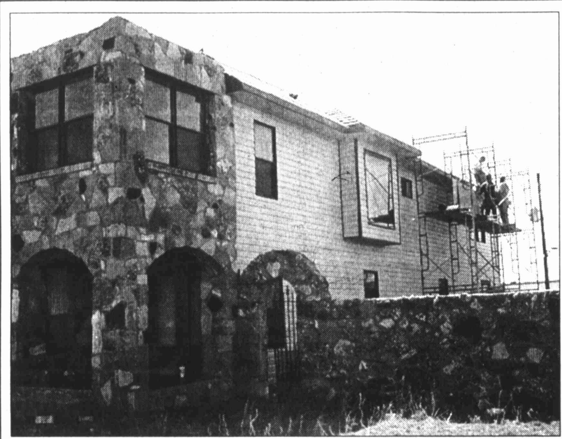
HERALD photo/Lyndel Moody Employees of J&M Construction work on the roof of this residence located on 1308 Scurry. The building is being remodeled and will be used to house unwed pregnant teenagers. Several area and national churches will be helping to renovate the home.
