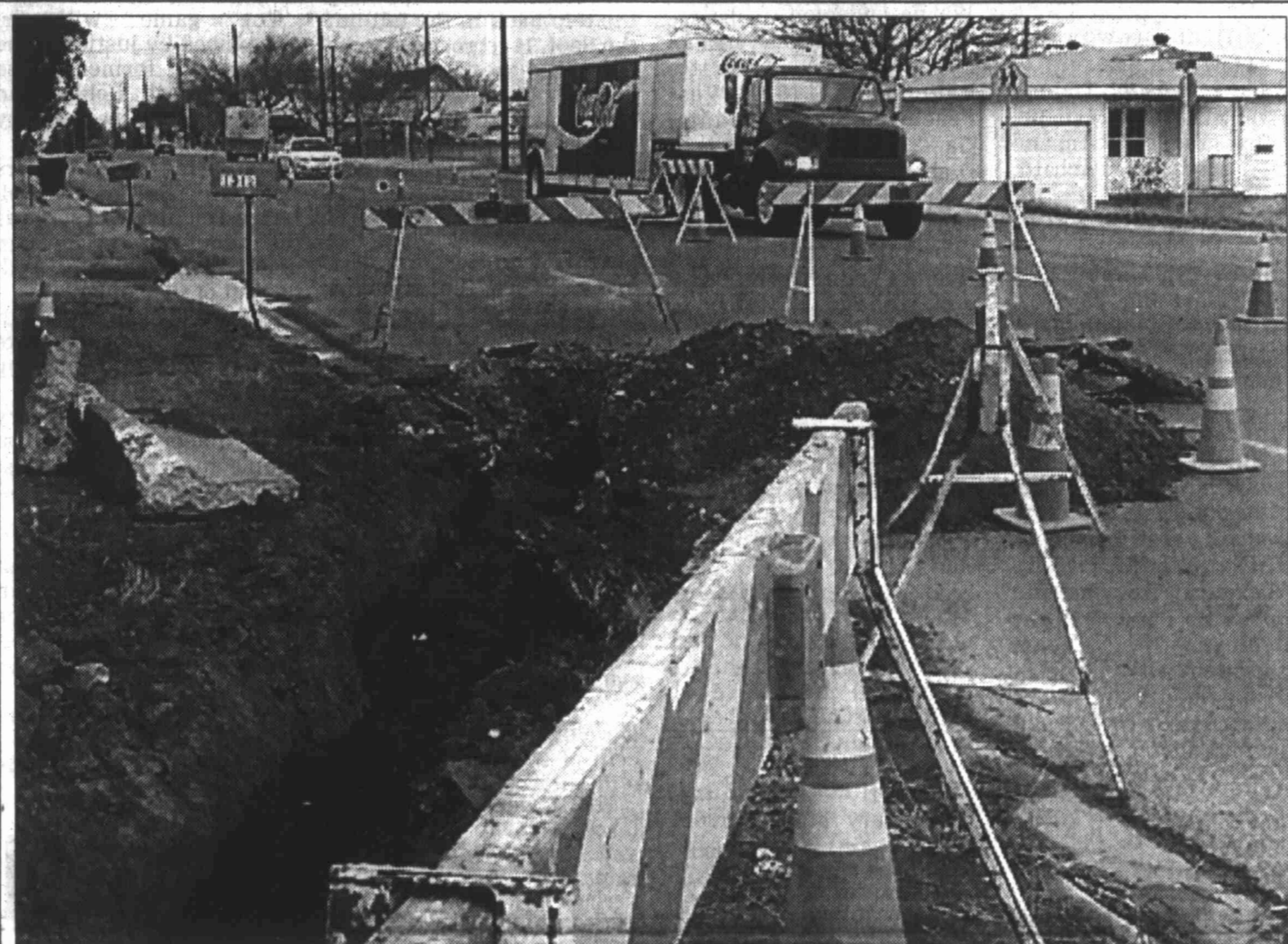
Traffic was diverted to two lanes on Birdwell Lane this morning after city of Big Spring employees dug a hole to work on a sewer line. The city was installing a new sewer tap for a house on the corner of 14th and Birdwell and expected to have the street fully opened by this evening.
