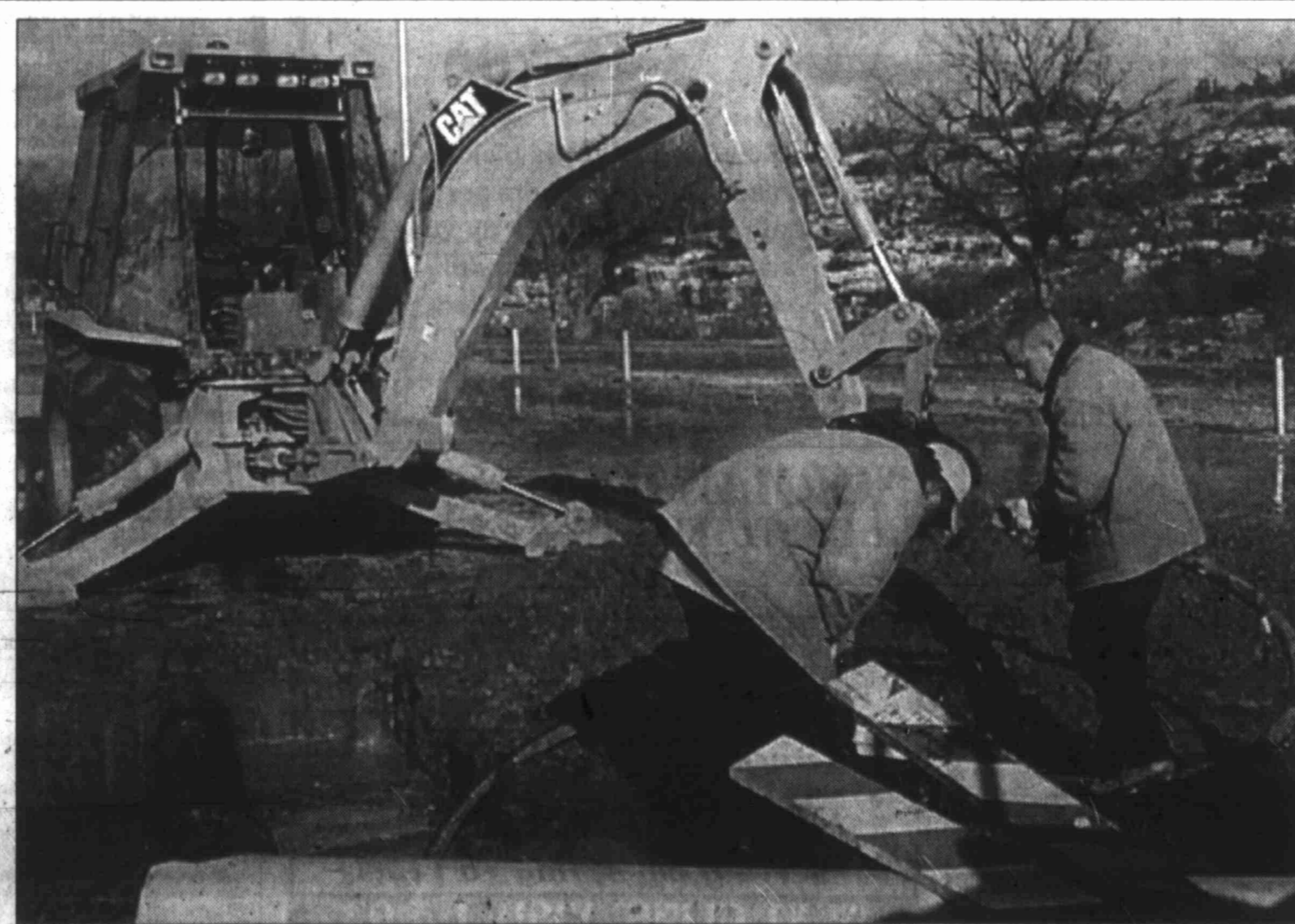
Jay Lopez and Cory Baker of the Big Spring Water Department set up a pump to drain water from around a leaky 12-inch water main Monday morning in Comanche Trill Park before they get down in the hole to patch the pipe.
