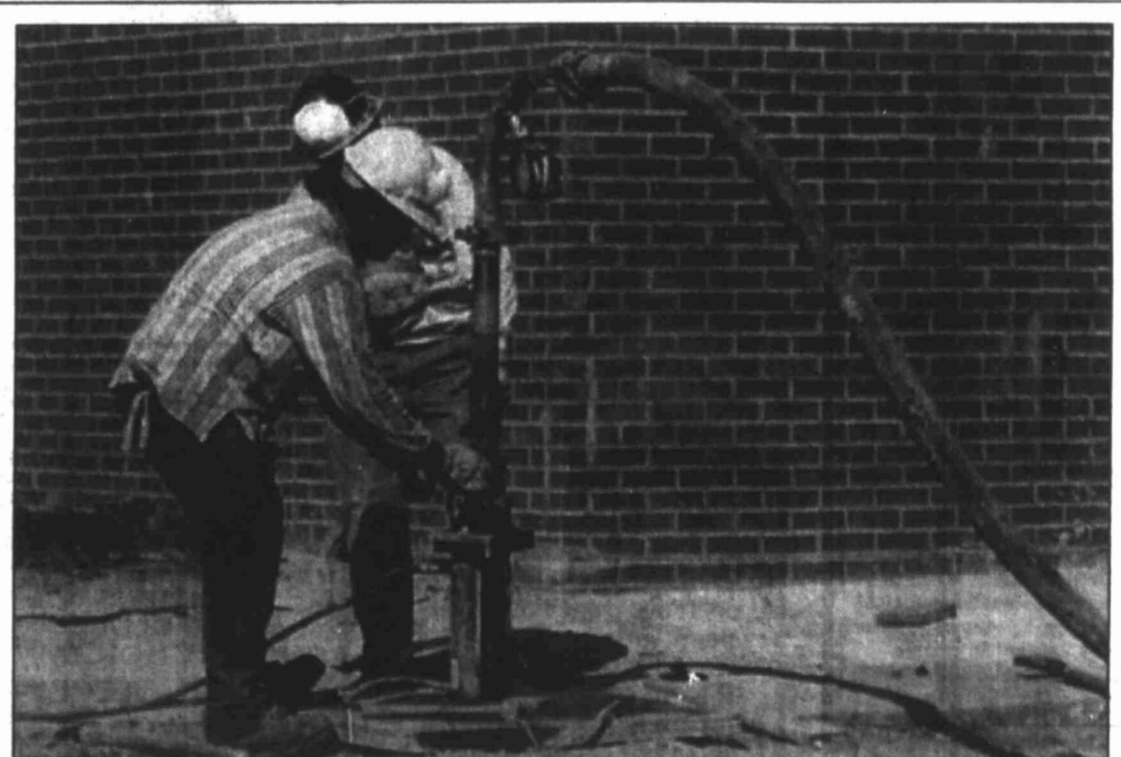
Richard Poucholoun, left, and Pedro Alvarez, both of Haywood Baker Grouters, secure the tube pumping concrete into the ground in an effort to expand the foundation at the Big Spring Junior High. The company is finishing grouting work begun in February to attempt to stabilize the building's foundation and expects to continue the project for at least two more weeks.
