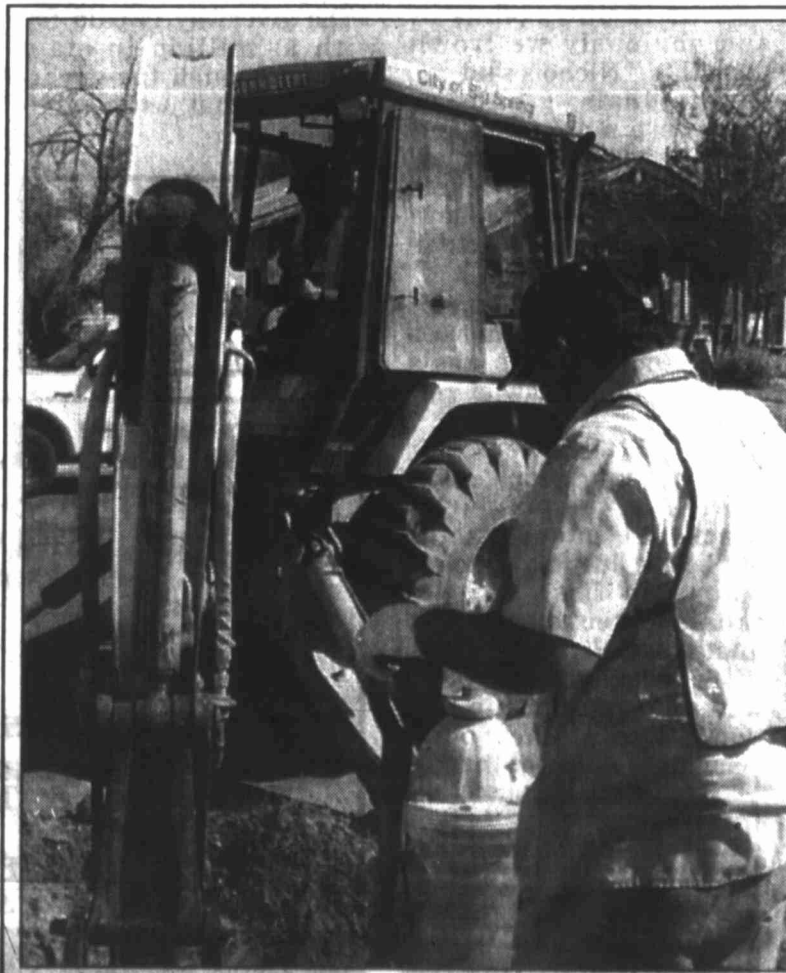
Backhoe operator James Darling and co-worker Andrew Martinez of the Big Spring Distribution and Collection Department work to remove and replace a fire hydrant at the corner of Third Street and Benton Avenue at about 10 a.m. today. The hydrant was due for routine replacement and had been "black bagged" by the D&C Department, indicating that it was out of service, said D&C spokesman Jim Piper. The workers had to shut off the water main in the area, so customers on Third Street between Austin and Owens Avenues experienced low pressure or outages.
