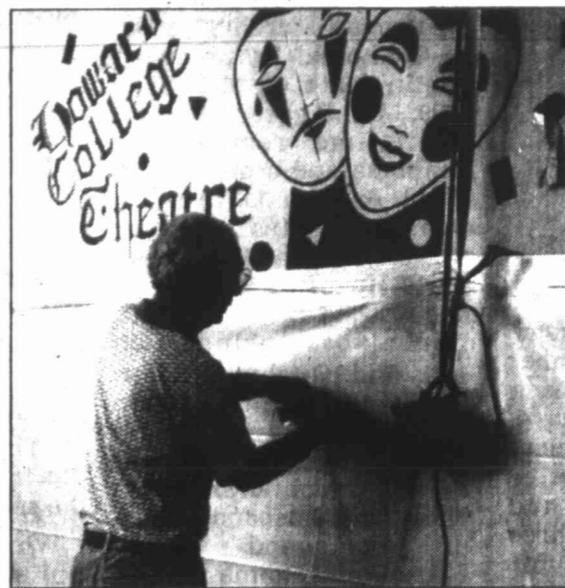
Doug Dallas, environmental specialist for King Consultants, checks a filter in an area where Texas Department of Criminal Justice inmates are removing asbestos material at the Howard College auditorium.
