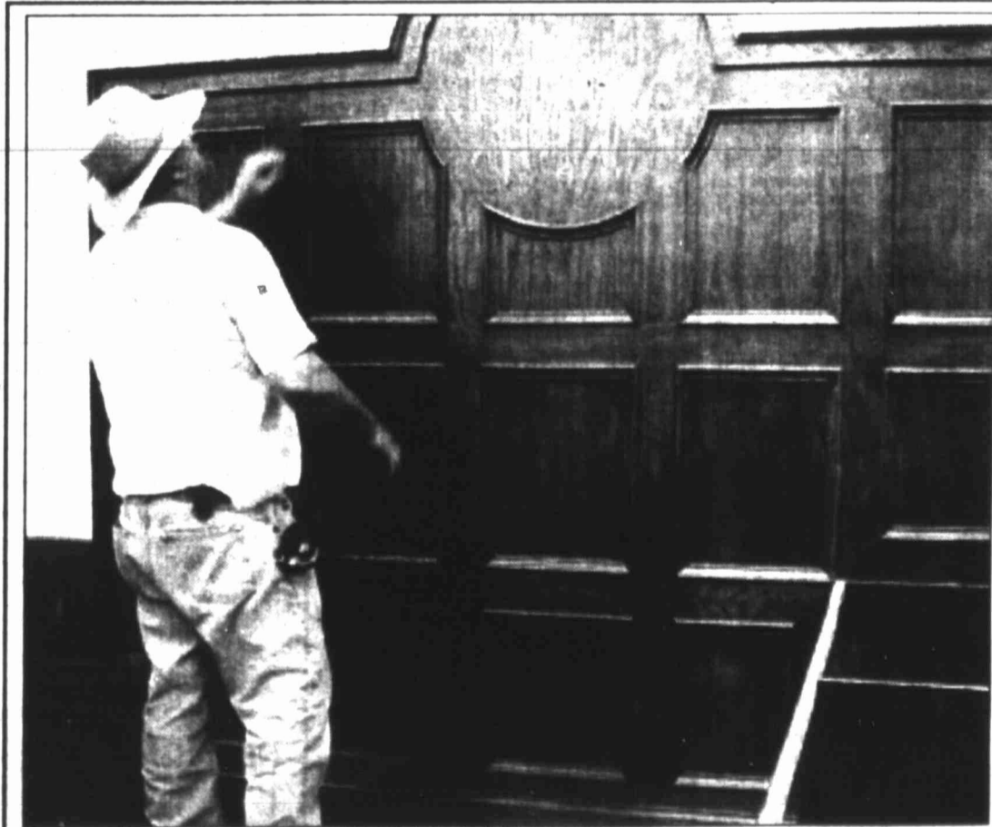
Project superintendent Pat Collins shows the backdrop behind the 118th District Courtroom bench. Renovation of the former Howard County Library into a district court building is set to be completed by the end of June.
