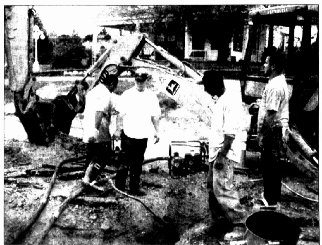
City of Big Spring crew workers were out Wednesday in force. From left, Mike Rivera, Randy Roach, Cody Rich and Johnny Gonzales replace a customer's service line at Eighth and Lancaster.
