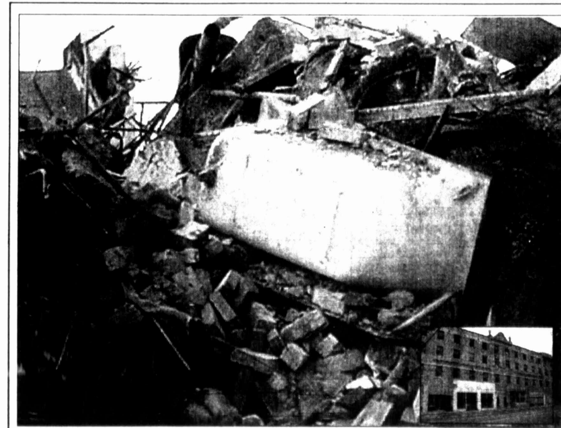
A bathtub was one of the few recognizable objects that remained in the rubble that was once the Howard House. Demolition of the building began last week and had been reduced to a pile of rubble by Wednesday afternoon. It could take weeks to haul off the debris, however. Inset — the Howard House prior to demolition.
