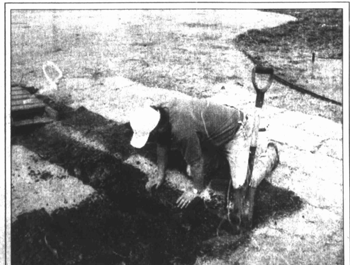
Richard Wright does some repair and replacement of the sprinkler system lines on the courthouse lawn. Some of the lines were recently damaged during some other work being done on some gas lines.
