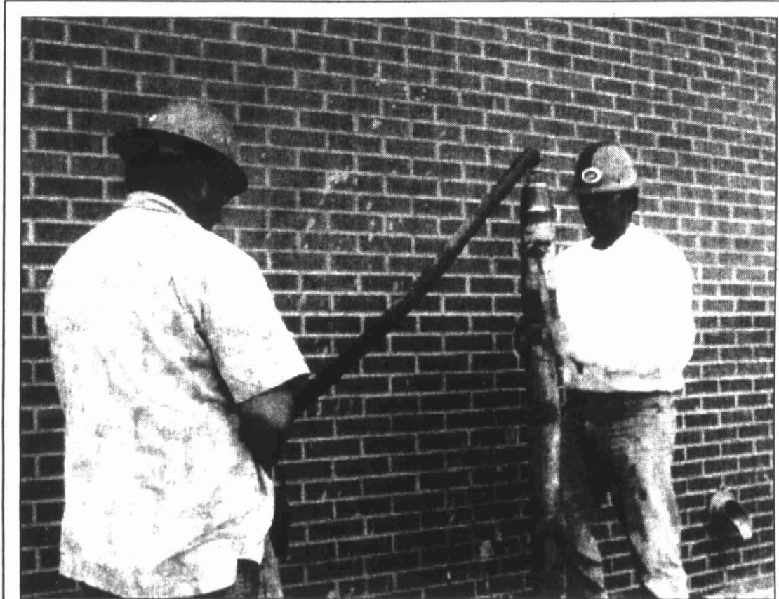
Hugo Mendoza, left and Mario Pouchoulen, employees of Haywood Baker Grouters, prepare to begin compaction grouting at the Big Spring Junior High School today. Haywood Baker was recalled to do additional grouting after a study showed the building continues to suffer foundation failure.
