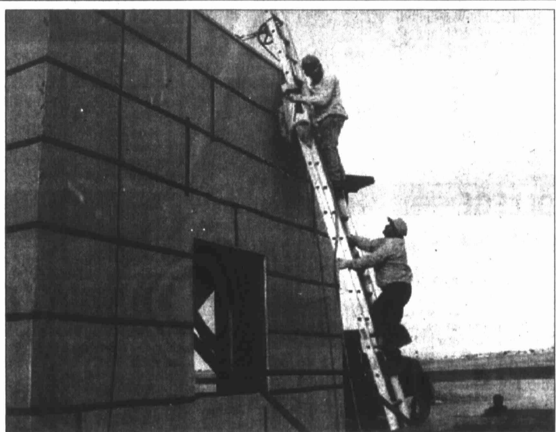
HERALD photo/Lyndel Moody David Clawson, left, and Emundo Martinez, both of Harrison Roofing, climb down from the roof of the McMahon-Wrinkle Airpark terminal after putting in insulation Monday. One of the agenda items for Big Spring City Council tonight calls for permitting Energas to service the soon-to-be-completed terminal with natural gas.
