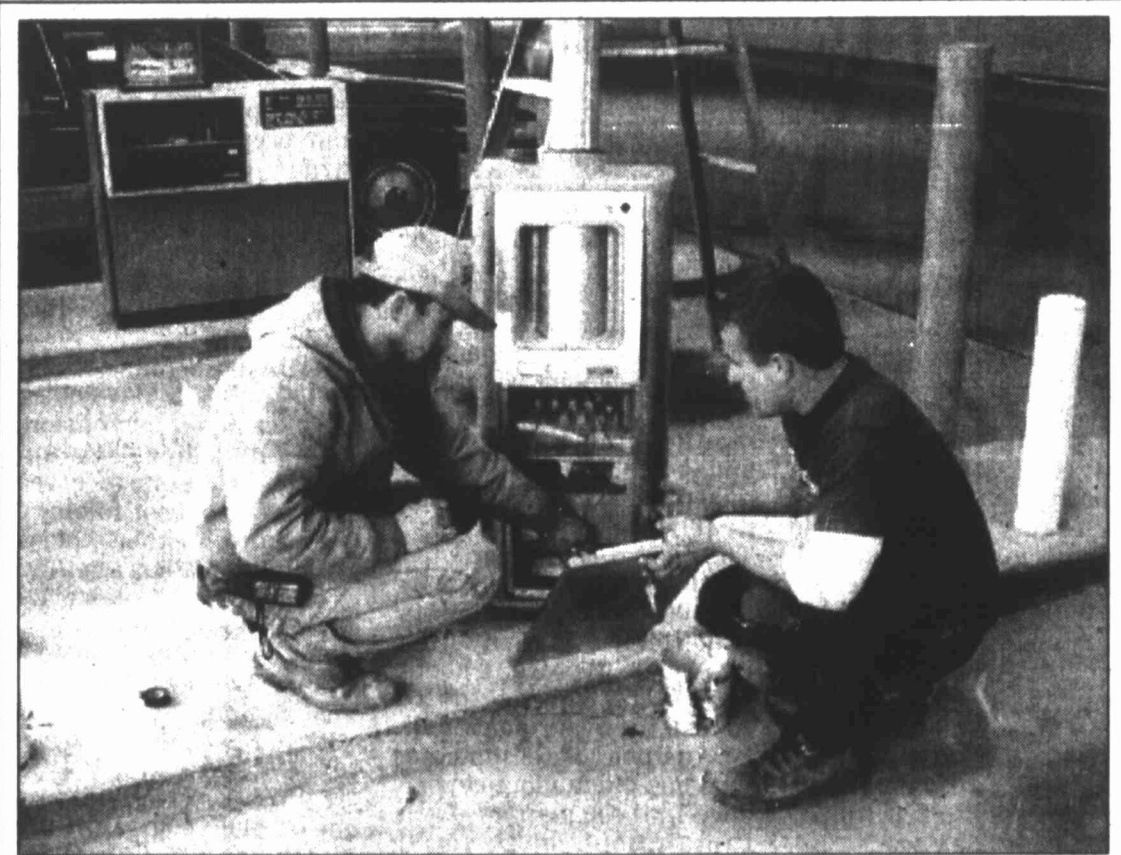
HERALD photo/Carl Graham Jason Slovak and James Brown of Security Vault Works of Dallas install new pneumatic canister chutes at Wells Fargo Bank. The machines should be ready to use by Tuesday.
