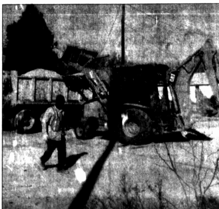
After throwing some trash in the dump truck, Cody Ridge of the distribution and collection department walks to the side so fellow employee James Darling can finish filling a hole made by workers to repair a waterline break. City employees worked round the clock to fix a rash of breaks scattered throughout Big Spring.
