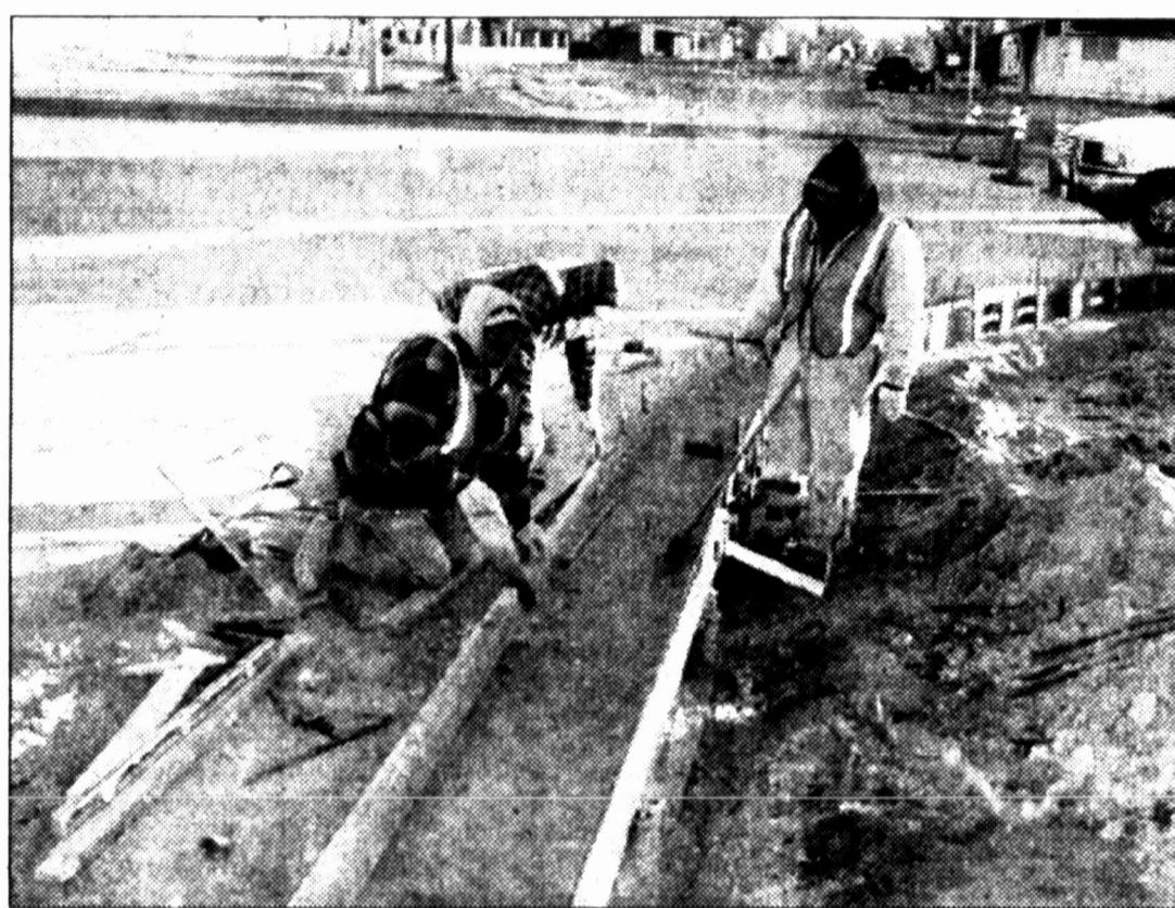
Reece Albert construction employees Elizondra Mascorro, Wemeslao Chacon and Sylvester Antonio prepare gutters for pouring concrete as construction continues along U.S. Highway 87 from Fourth Street to Interstate 20.
