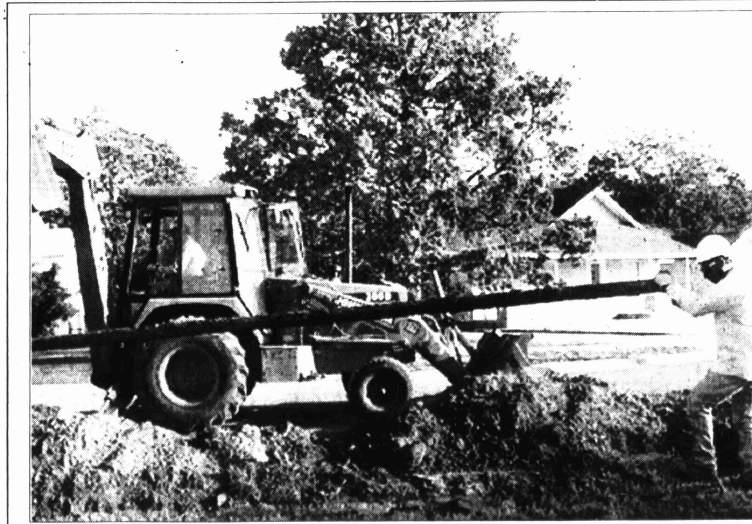
Energas employees were replacing a 50-year-old natural gas pipe that had developed a small leak in the 100 block of Lincoln this morning. Senior construction operator Pete Garcia balances the pipe as it is lifted up from the ditch.
