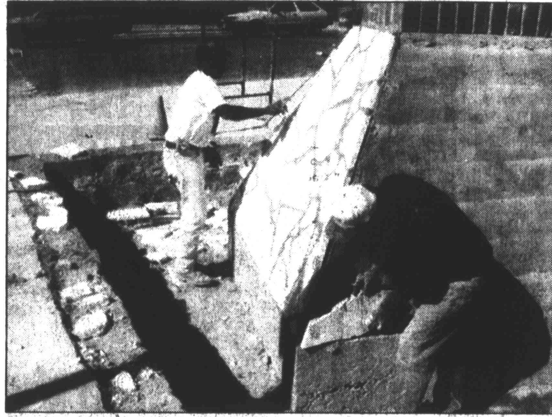
Thomas Lewis, left, and Riley Faulkner of Faulkner Masonry work on a new sign being constructed for Moore Development for Big Spring and the Big Spring Area Chamber of Commerce. The sign, a joint venture between the two entities, should be complete in a week to 10 days.
