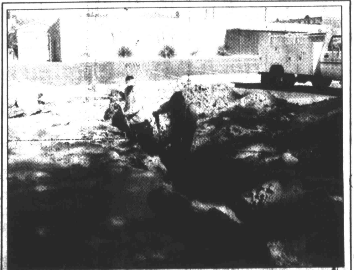
City workers Chris Martinez and Jennifer Dubose prepare to put in a new line at 808 Scurry, the new location of the United Way of Big Spring and Howard County. The building is also occupied by the Big Spring Symphony Association. 1 Guild.
