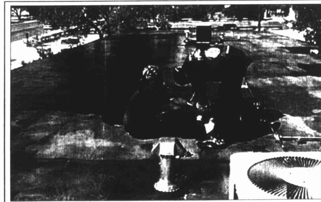
Proffitt Day Care Center will re-open at 6 a.m. Thursday with a new roof. The roof was blown off in last Sunday's thunderstorm. B&M Roofing employees Jerry Garcia and Tim Reed are shown working on their tar machine. Pinner Carpet of Odessa donated new carpet to the facility after hearing of the plight on an Odessa television story.
