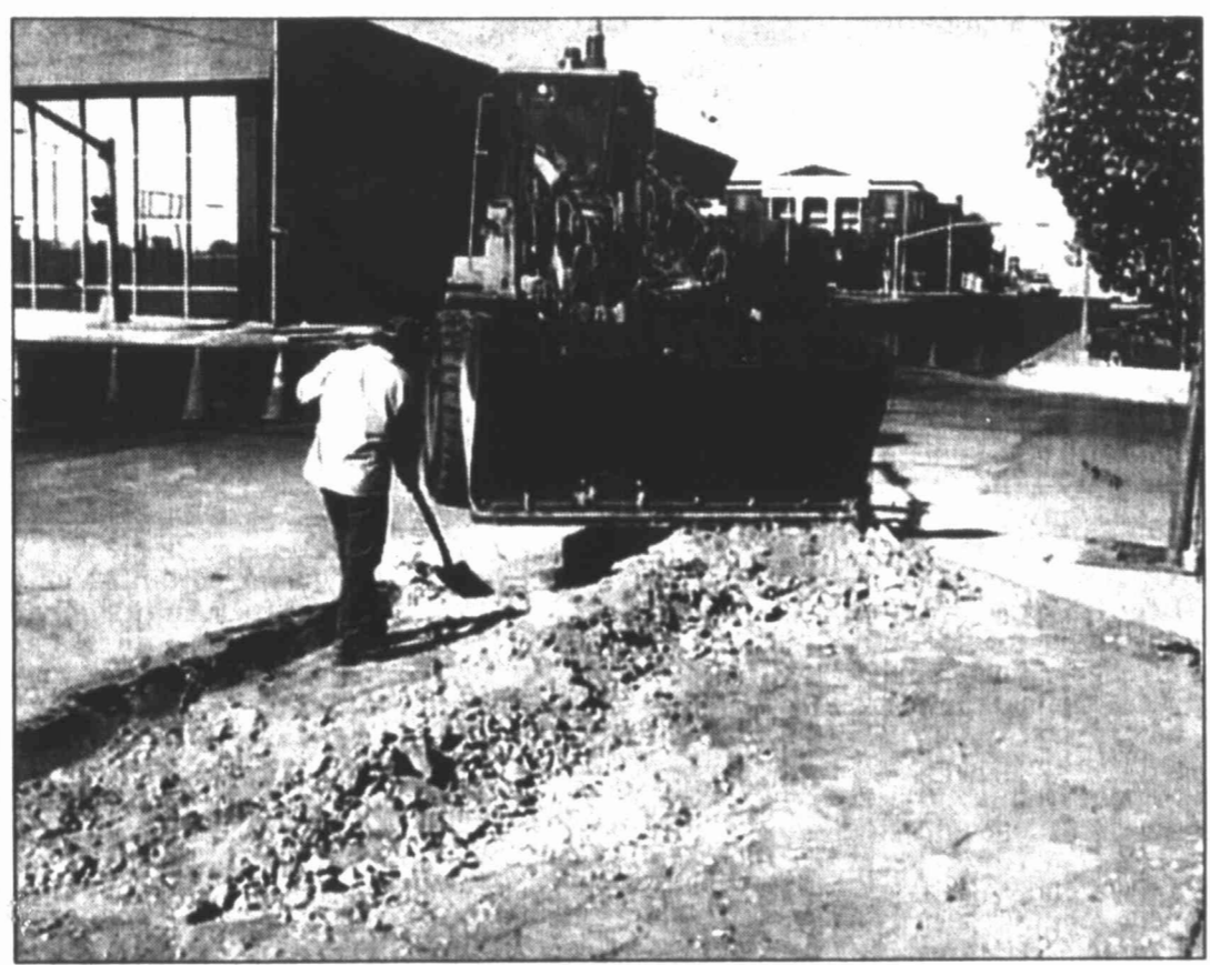
HERALD photo/Carl Graham Rual Martinez of the Big Spring city street department shovels concrete so that Jorge Parra can take it away from the sidewalk. New sidewalk will be replacing the old near the courthouse at Third and Main. Work is expected to last several days.
