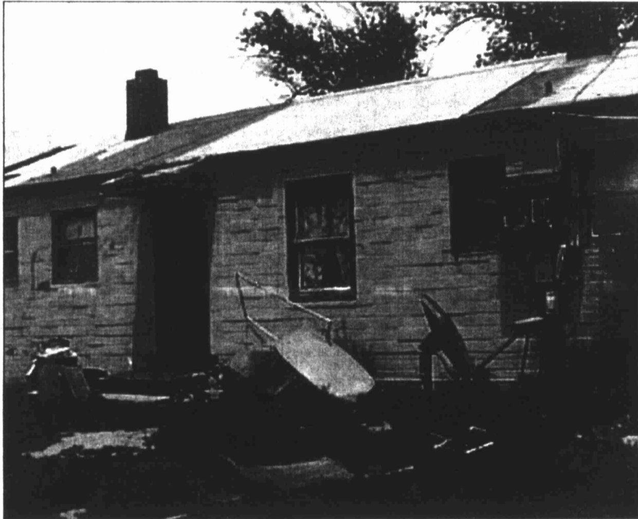
At least 11 units at the Apache Bend apartments are currently rented to tenants, city officials say. The complex at 120 Airbase Road was recently declared an unsafe building by the city's code enforcement office. The dilapidated structure, shown here from the back of an apartment on the west side, has numerous problems, including leaking roofs and infestations of pests, tenants said.
