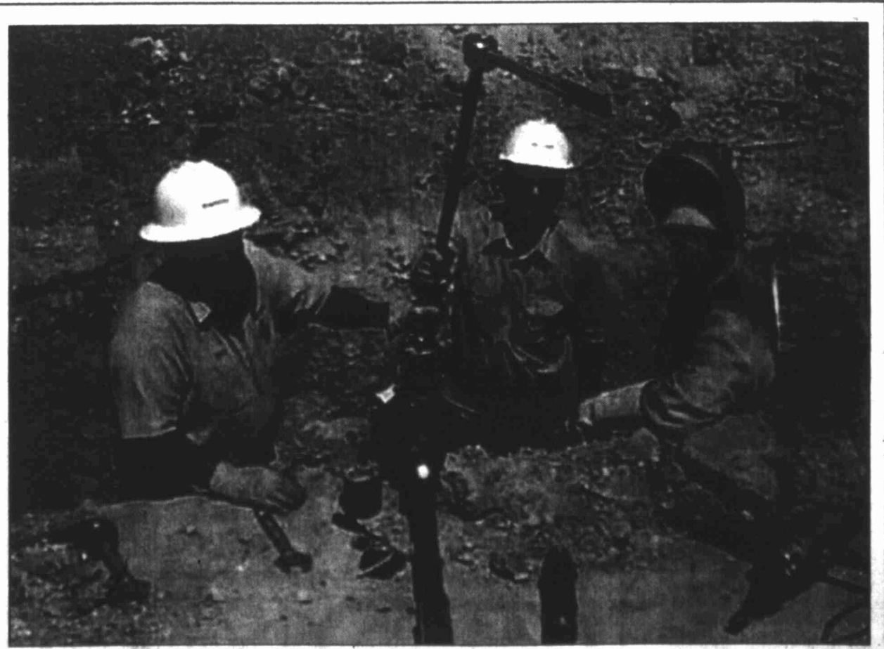
Energas employees Manuel Baeza, Richard Nix, and Rick Clark test for a gas leak that was reported at 207 West 17th. The crew located the leak and was able to take care of the problem.
