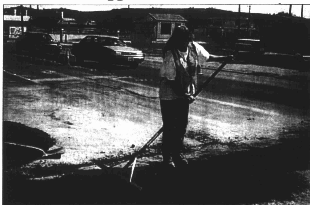
Jennifer Dubose covers a section across Gregg Street that was cut away, allowing city workers to lay new waterlines. The work is being done in preparation for extensive reconstruction project this summer.
