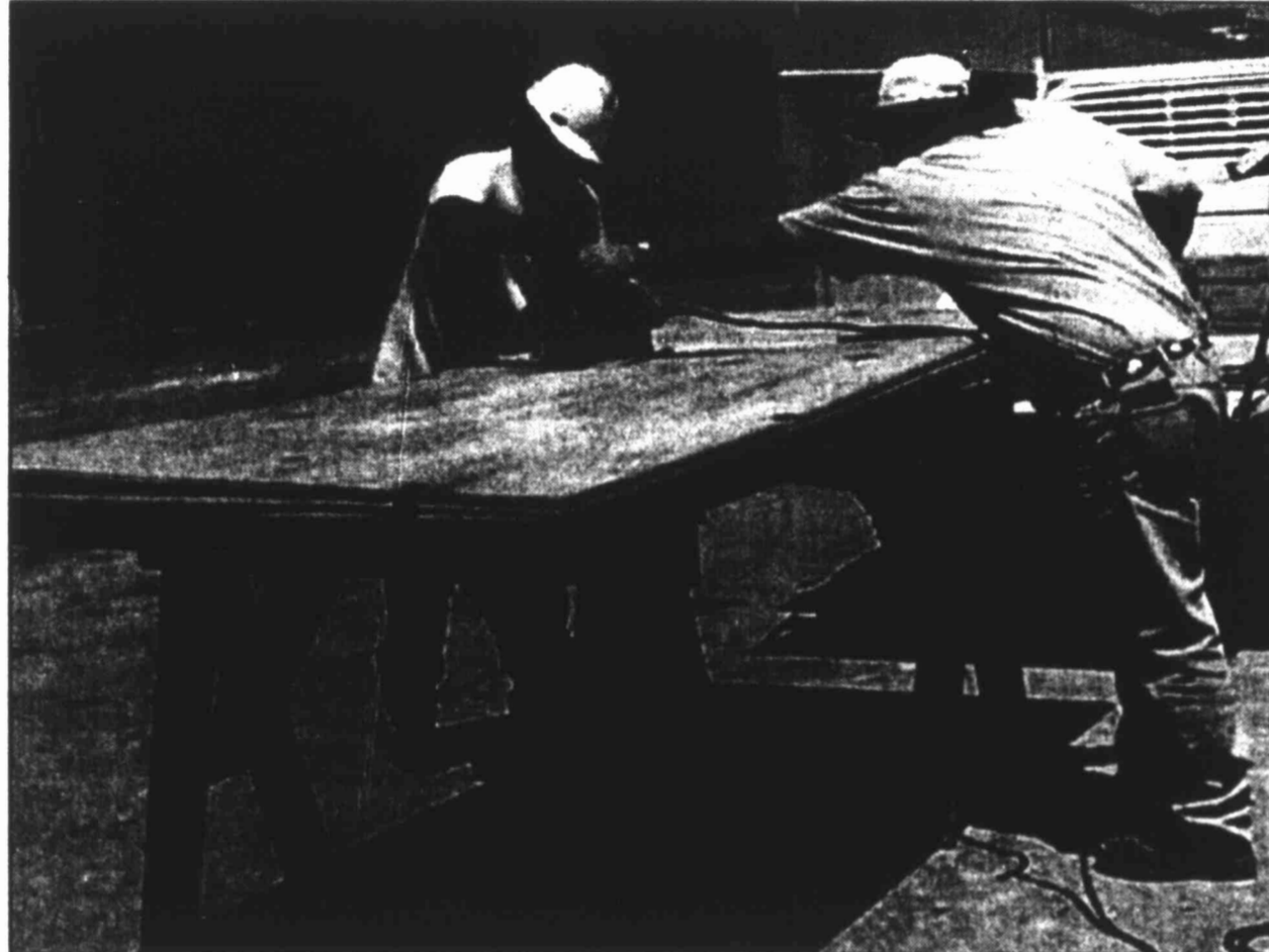
Ace Merrick, left, and Bob Menges cut wood panels to cover the window vents on the Western Container building. Western Container has a plant in Houston, Hattiesburg, Miss., and two in California. Nation wide, employees are about a total of 620, with about 180 being employed by the Big Spring plant. The Big Spring plant is the oldest Western Container plant.
