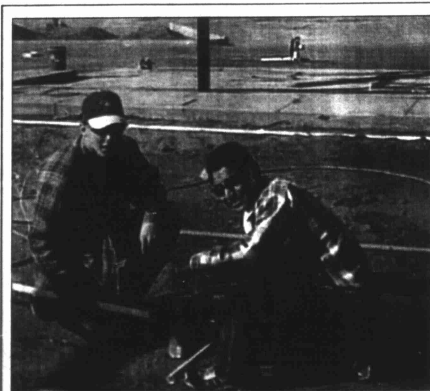
Johansen Landscape & Nursery workers Jeremy Green and Manuel Arriaga are installing irrigation lines for the new Sonic-Drive In on FM 700. Construction continues at a fast pace and burgers and fries will be served up in a few short weeks.
