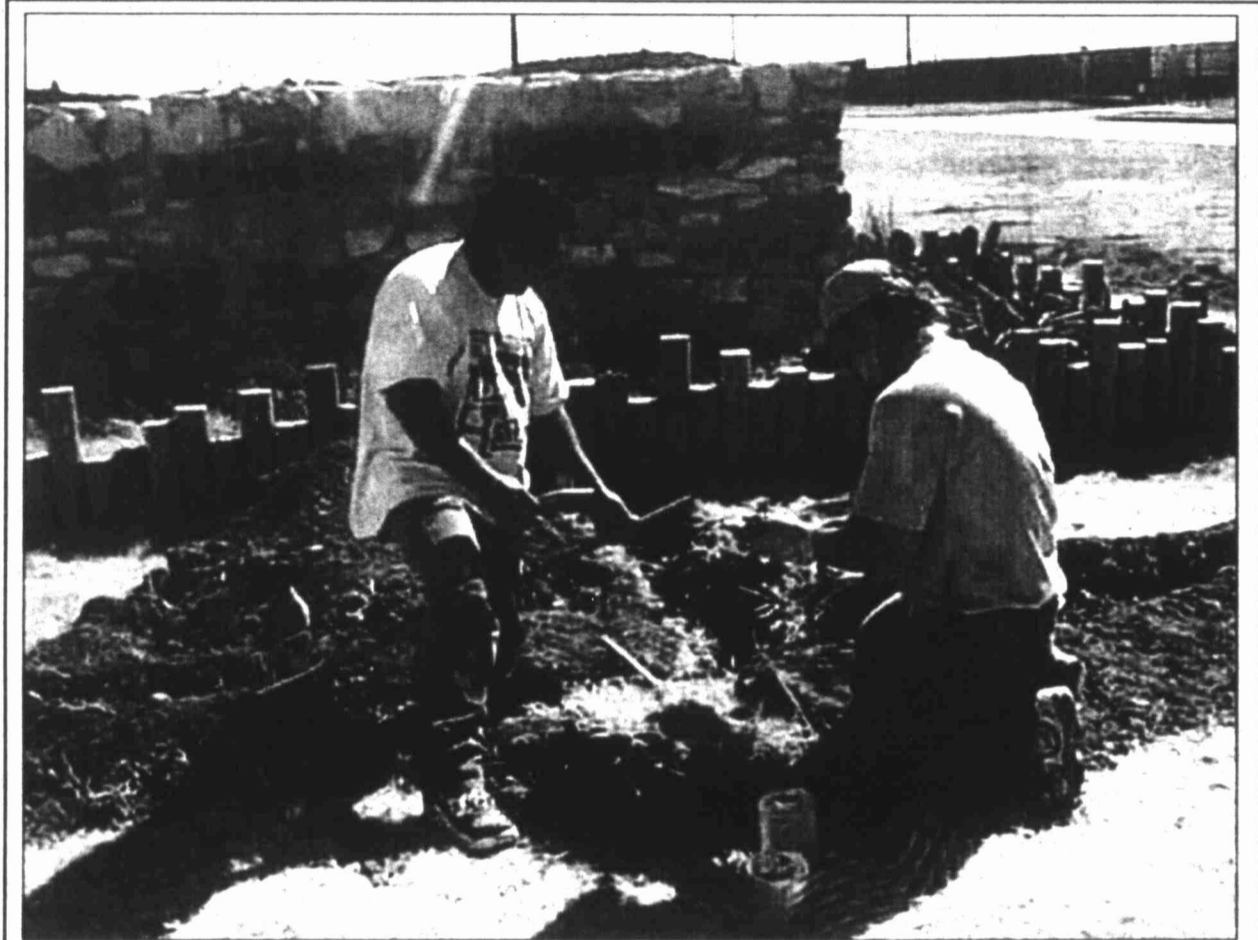
SouthWest Collegiate Institute for the Deaf maintenance crew members David Yanez and Brad Lentz busy themselves putting in additional lights on campus.
