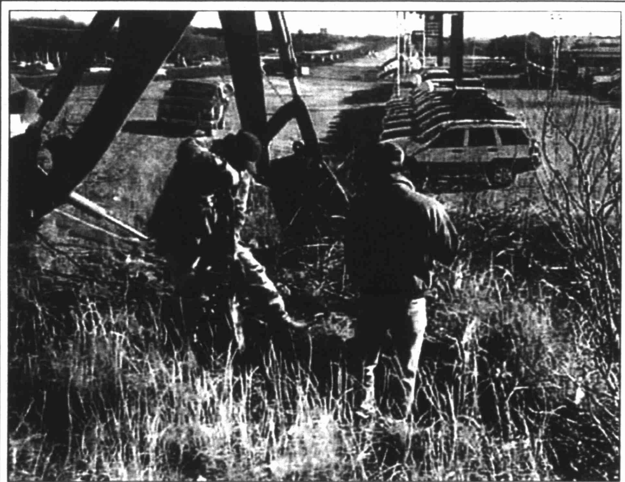
"Sluggo" Martinez and Steve English of Cline Construction are busy digging up buried cable for Southwestern Bell telephone company. The work is being done next to Fiesta Dodge in the 500 block of FM 700.
