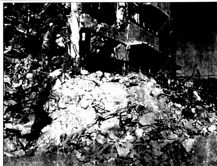
Rubble from the Permian Building is being used to fill in some low places around the city and prevent erosion. The county has provided equipment to assist in the project. Midwest Wrecking is demolishing the old building and hauling the debris to the fill-in sites.
