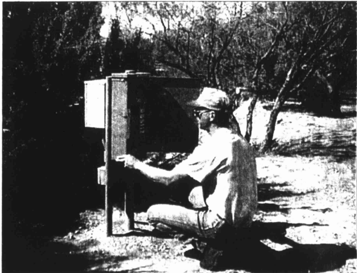
Dana Duncan, committee volunteer for the Comanche Trail Festival of Lights, looks over a new electrical outlet that was installed in the park recently. Thanks to hours of work by contractors and volunteers, there will be three times as much electricity available for the lighted displays this year compared with last year.
